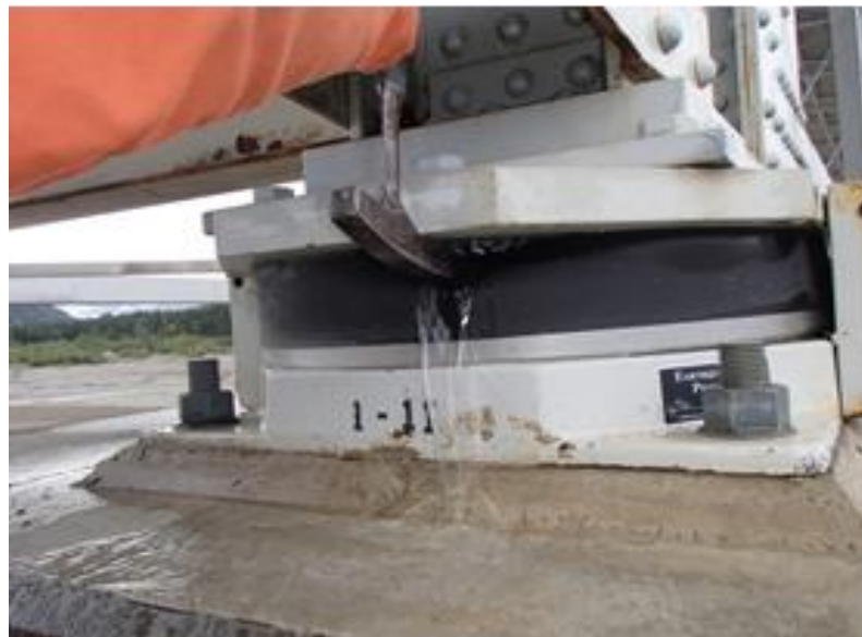
Figure 1.3. Water contamination in Alaska bridge (Alaska DOT, 2019)
