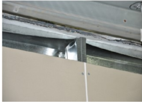
Figure 2-4: Lateral movement of stud from the top track on slip track partitions (Soroushian et al. 2016).
