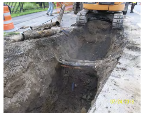
Direct bury electrical cable
