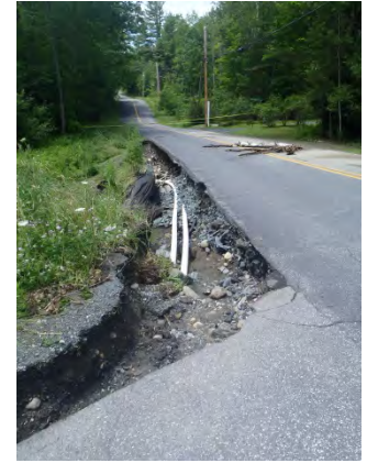
Washout from storm
