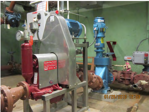
New Primary Sludge Pumps
