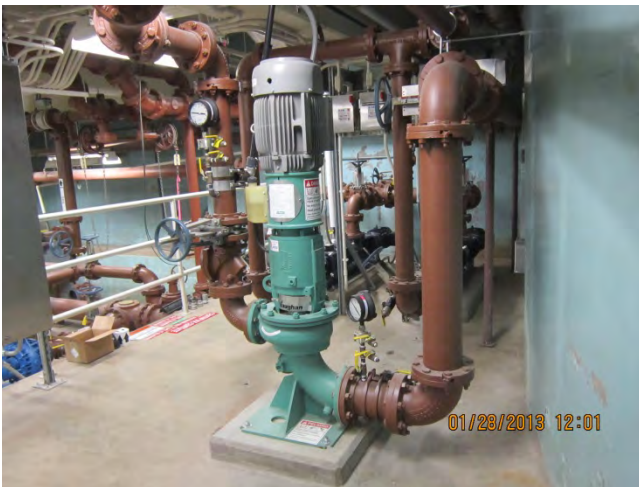
New Digester Recirculation and Transfer Pumps
