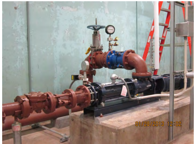
New Centrifuge Feed Pumps
