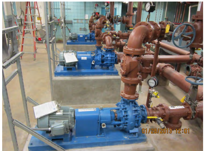
New RAS / WAS Sludge Pumps
