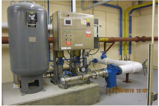
New Plant Water System
