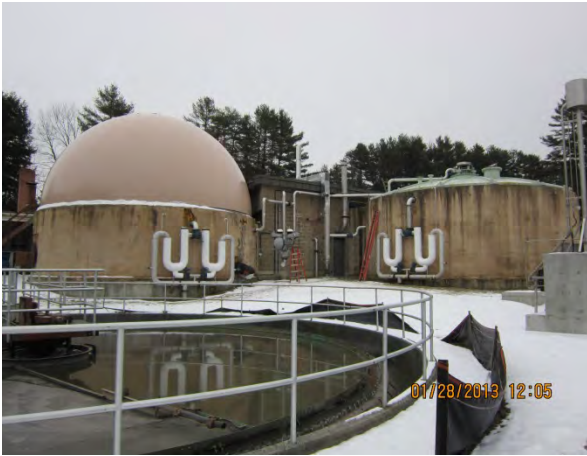
New Digester Covers and Methane Collection
