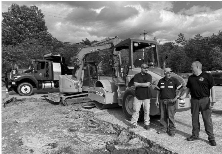
Repaving the central Fire Station parking lot with Ty Bryant, Jon Peaslee, Ted Call.
