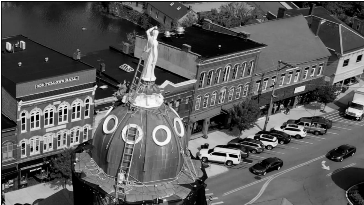
Exeter Town Hall repairs by Limerick Steeplejacks, Inc. Photo by Morning Star Aerial LLC.
