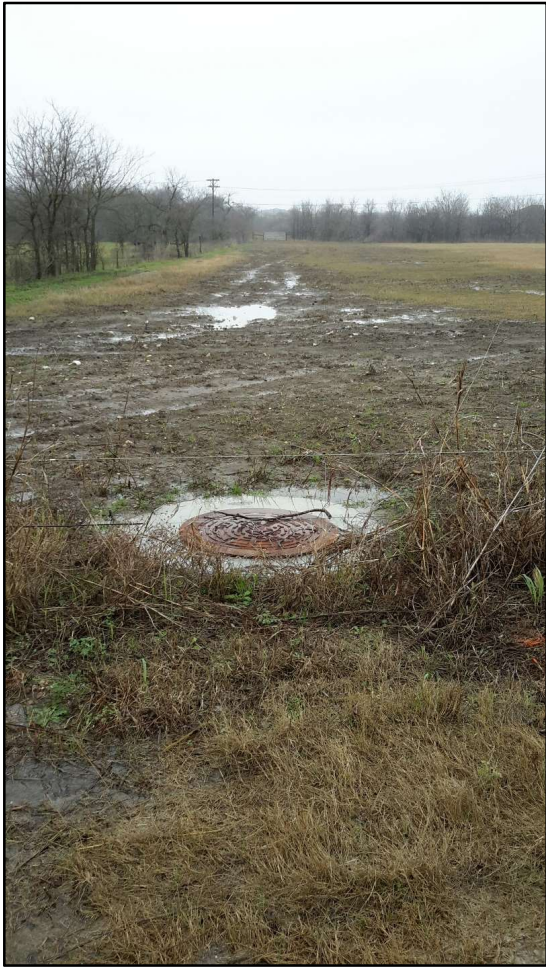
Figure 8. Recently installed wastewater line on northern end of project area, facing west.
