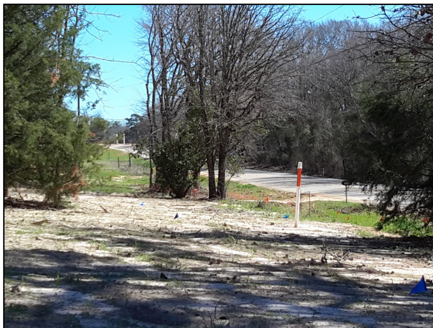
Figure 19. Heavily graded and disturbed proposed ROW with numerous marked fiber optic and water utilities typical of parcels near the Toll 49 construction area, facing southeast on parcel 57. Note that columns for Toll 49 can be seen in background.
