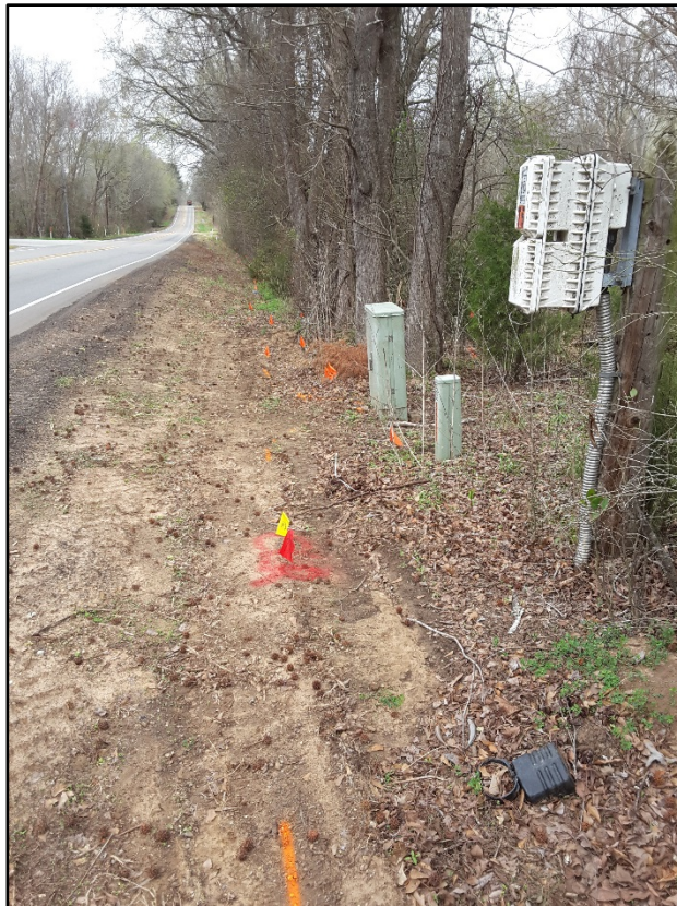
Figure 9. Numerous buried and marked utilities on edge of existing TxDOT ROW, facing northwest.
