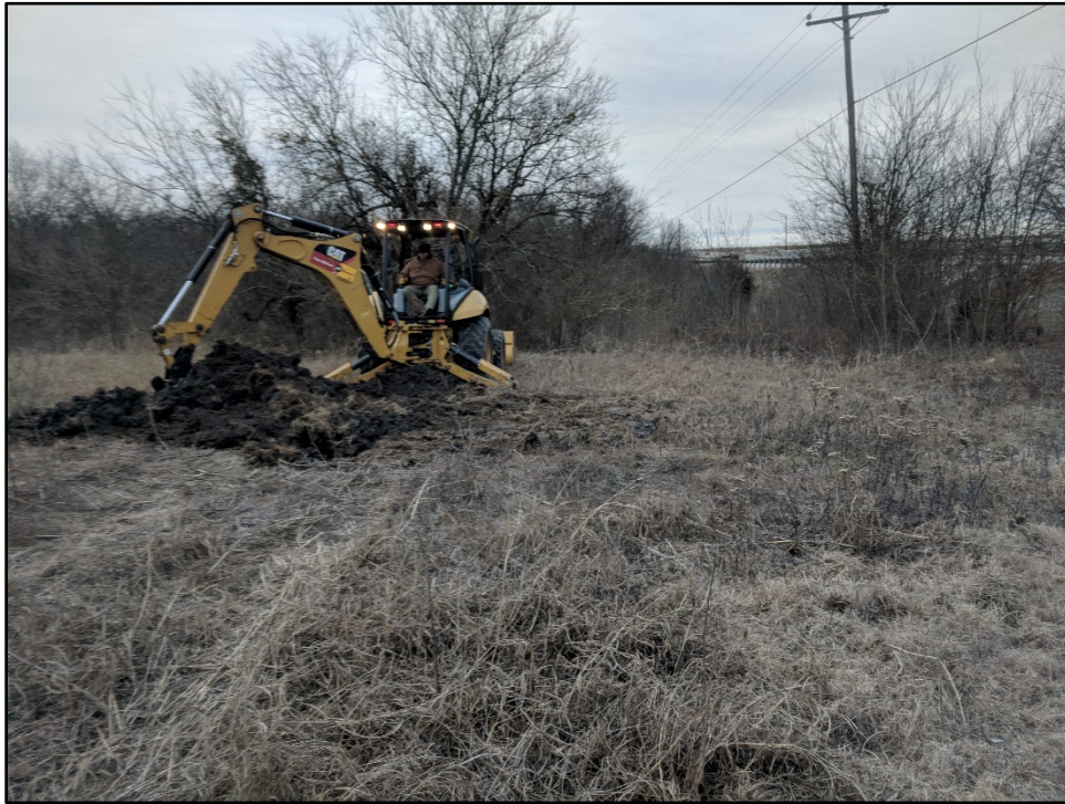
Figure 7. Overview of BHT 8 being excavated along the existing FM 148 ROW, facing southeast.
