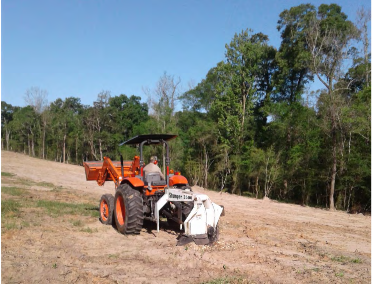
Figure 7. Tree stump grinding was carried out to preserve high value deposits identified during MAC data collection at 41LB42.
