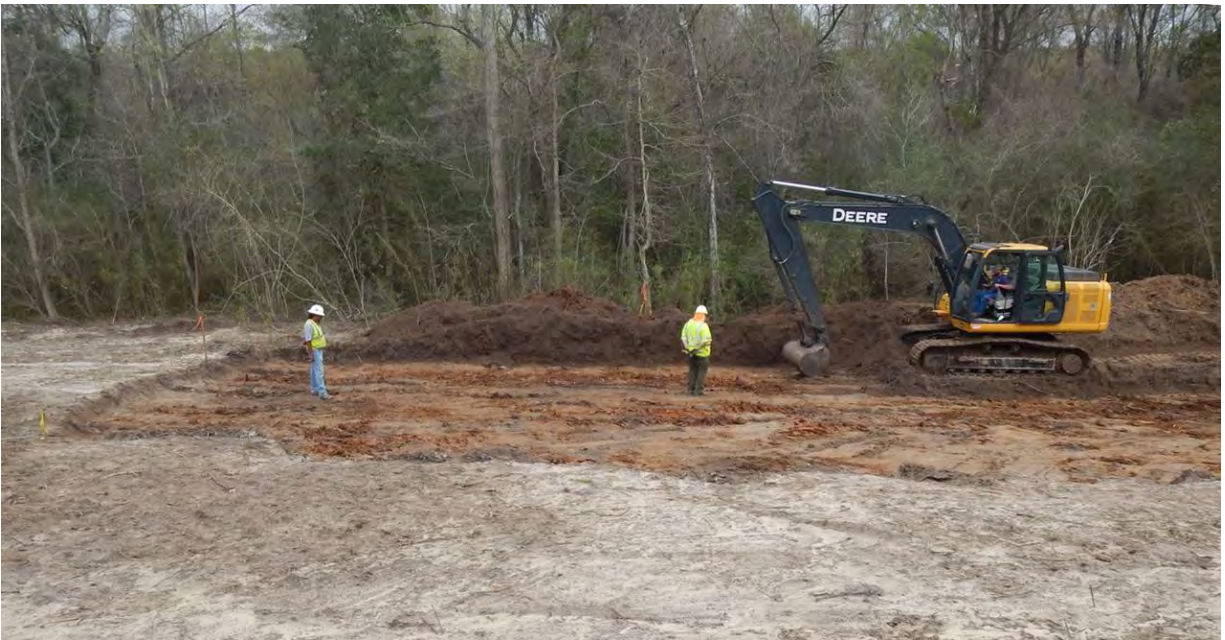
Figure 6. Mechanical excavations of pipeline ROW within 41LB42. Above facing east, MAC data recovery excavations were located near the vehicles in background. Below facing north.
