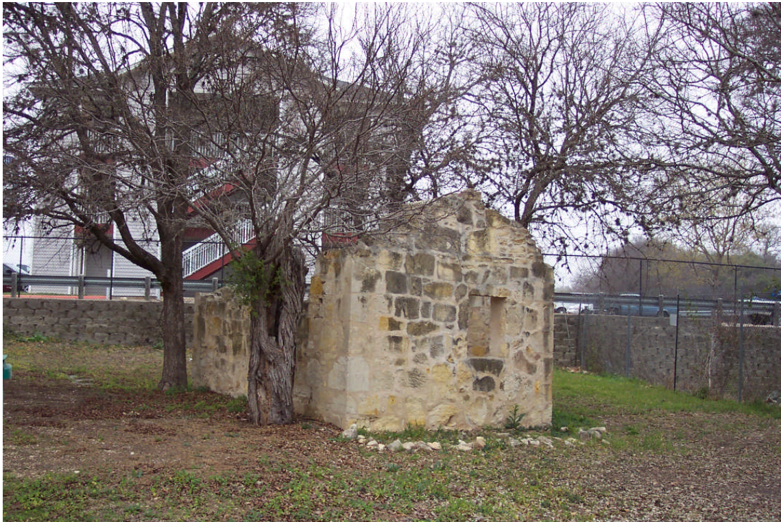
Figure 3. View toward north of south facade of kitchen (ruin) behind Huebner-Onion Homestead house. Note proximity of motel to north and east of historic site. Taken by Imogen R. Cooper on March 1, 2014.
