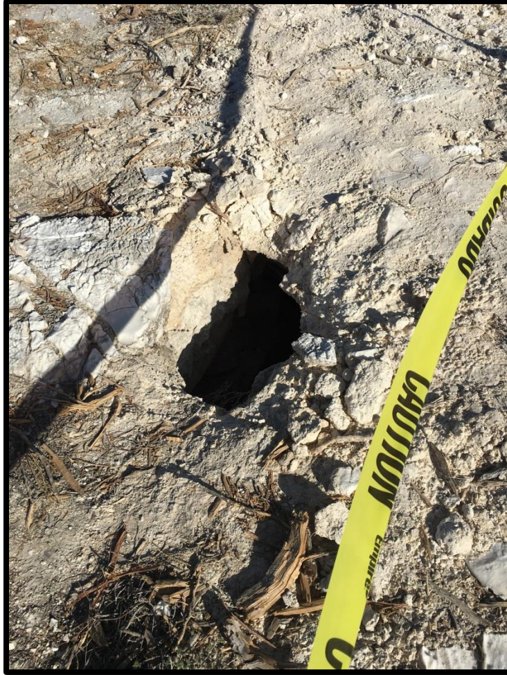
Figure 76. Small Vertical Cavity to the North of Main Cavity, Measuring 44x33 cm
