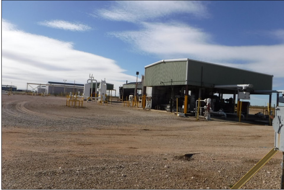
Figure 2.1 Station No. 142 overview looking southwest
