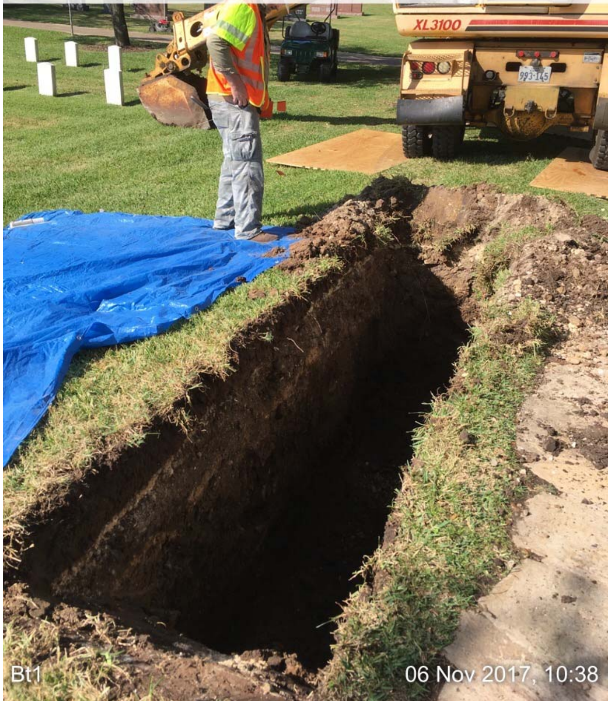
Figure 6: View of GT1 after excavation, showing the minimal impacts to the surrounding landscape.
