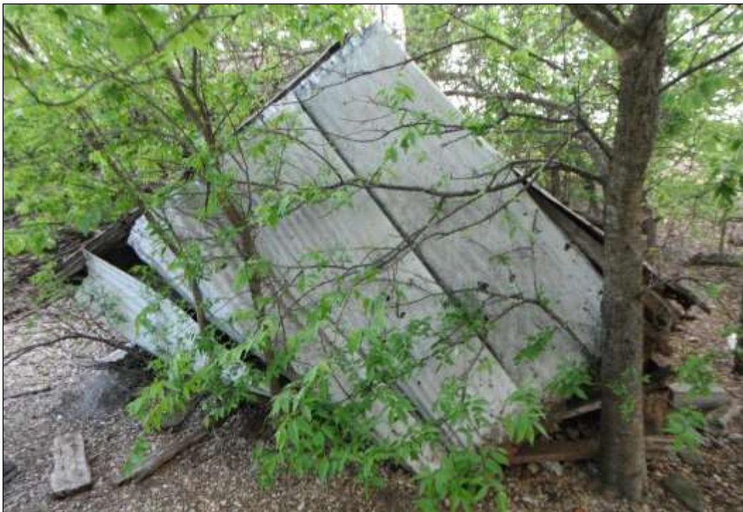
Figure 6-65. Structure W6-B (41HY541)—Collapsed Shed (Facing South)
