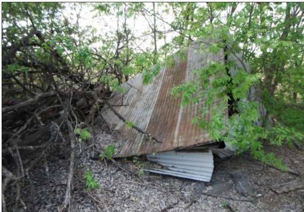
Figure 6-66. Structure W6-B (41HY541)—Collapsed Shed (Facing West)
