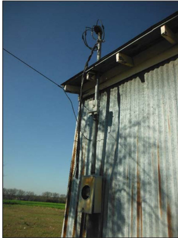
Figure 9. Electrical box at southeast corner of Feature 1 at site 41COL269. View to southwest.
