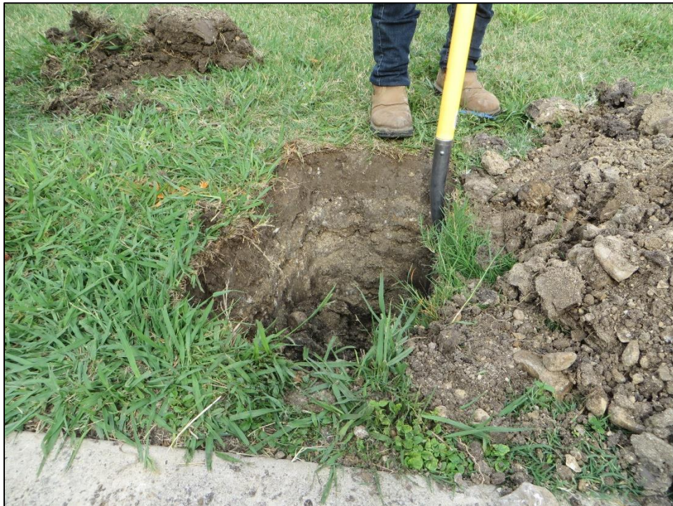
Figure 7. Overview of the excavation of BP 1 and west wall profile; facing west.
