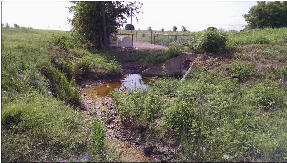
Photo 7. Southern end of alignment. Note disturbances from lift station and roadside drainage. View to the east.
