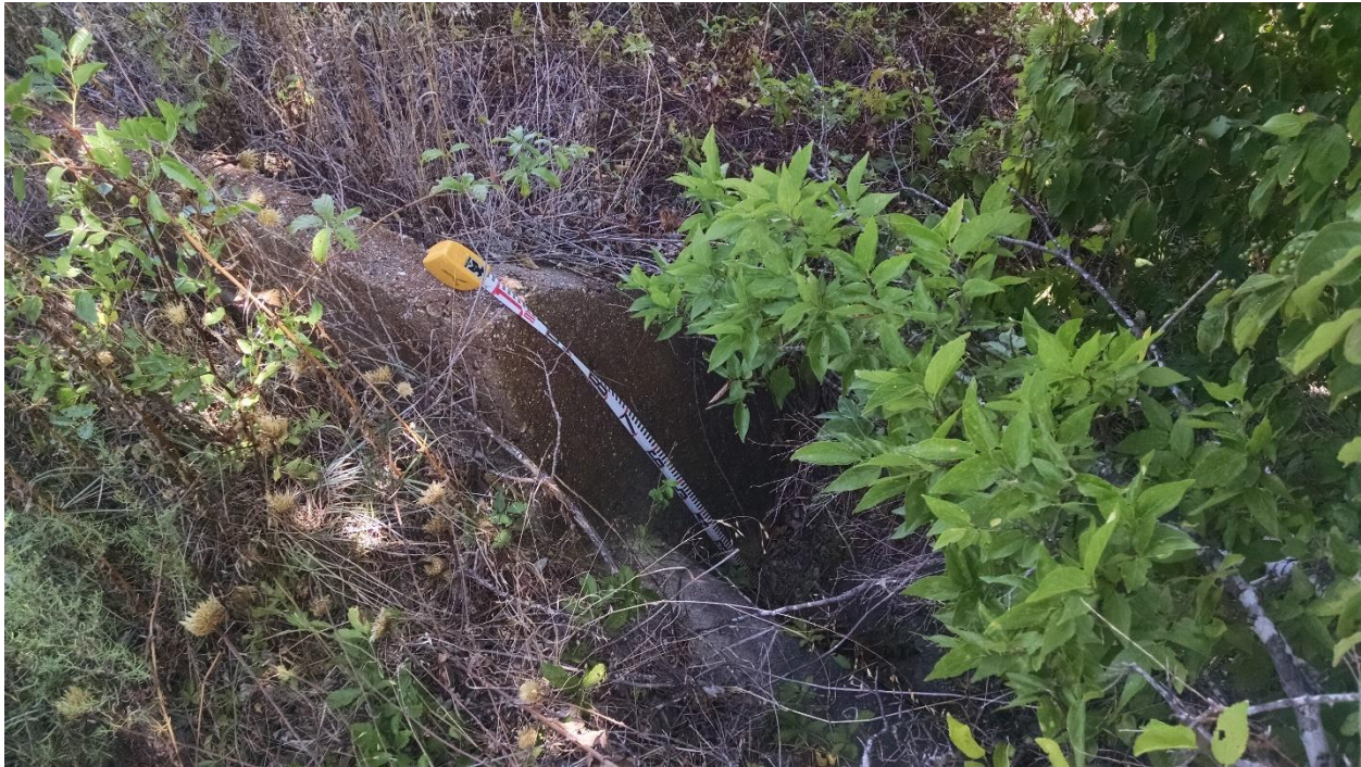
Photo 11. Side view of isolated concrete agricultural drainage feature.
