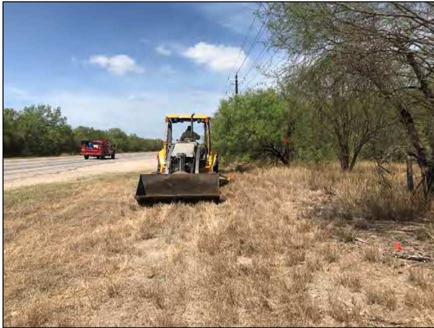
Figure 14. Overview of 41MC372 prior to trenching, facing west. Note informal pull-off area beyond backhoe and buried fiber optic line along fence line.
