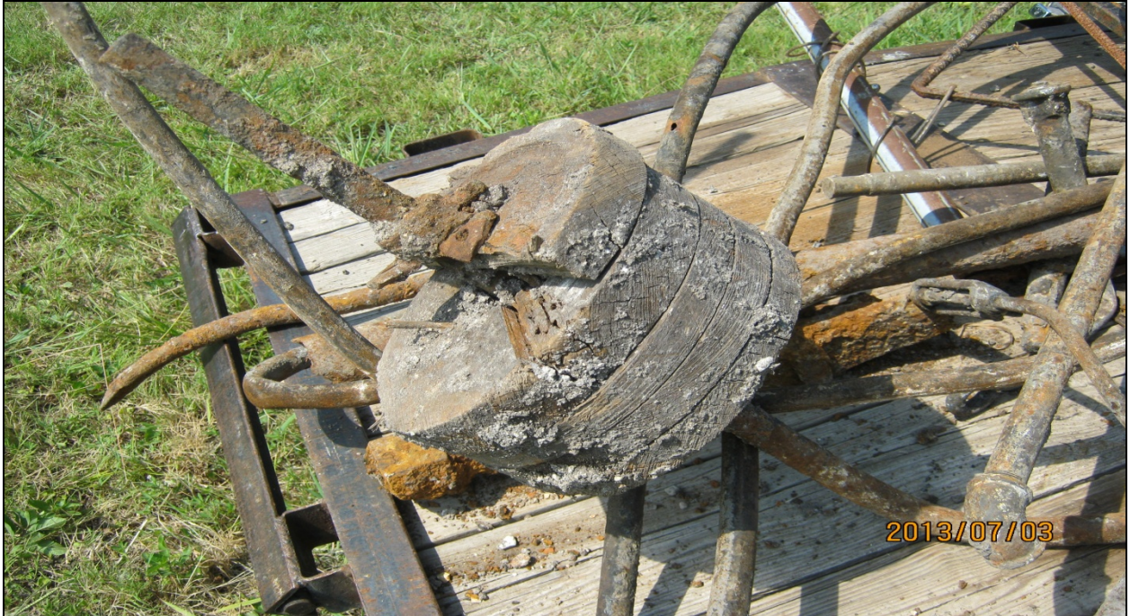
Figure 2. Pipes and internal components discovered during impact trenching of original dam wall prior to AAG monitoring the construction.
