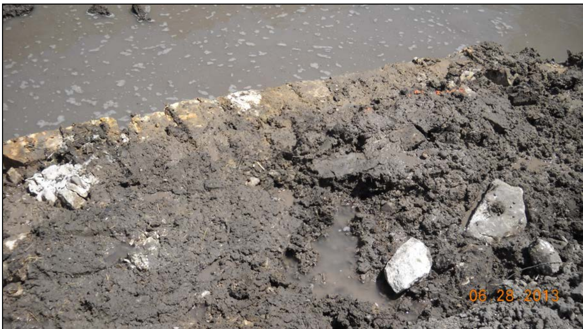
Figure 8. View of the remnant limestone wall from Gan's Dam.
