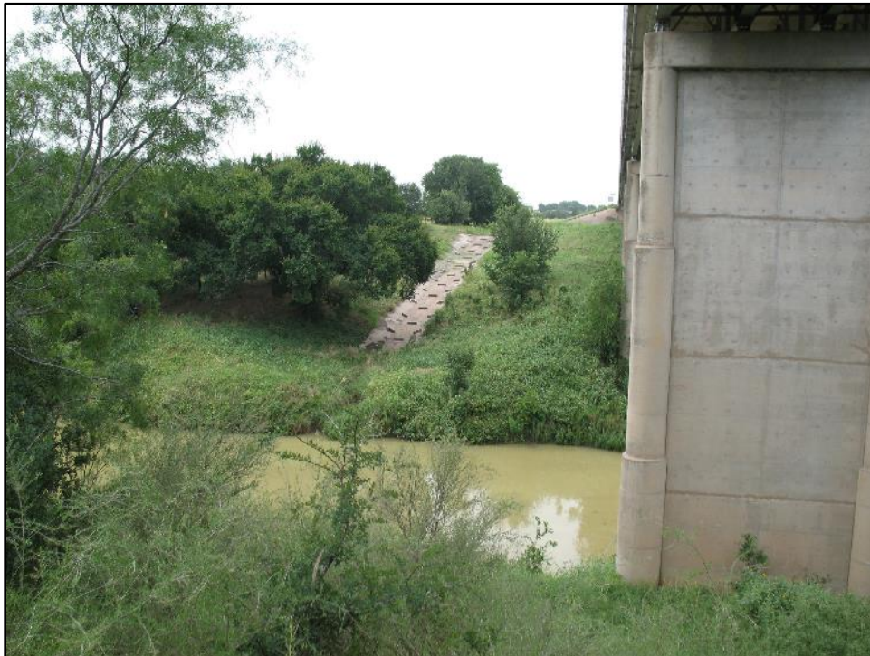
Figure 6. Colorado River and FM 45 bridge with road fill and added drainage features, facing south.
