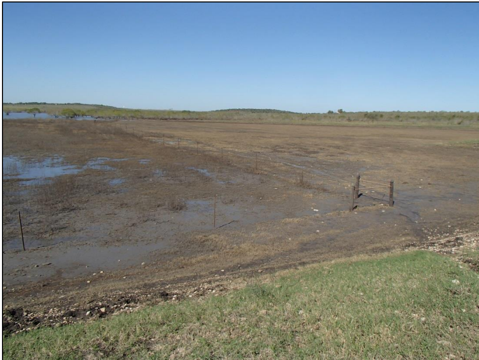
Figure 18. Eroded and devegetated drawdown area at north end of LOC within the auxiliary spillway. Facing north.
