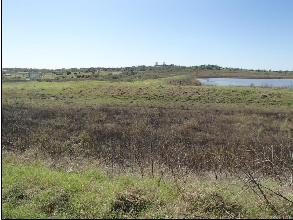
Figure 9. View of disturbed auxiliary spillway area in foreground, and earthen dam in background. Facing southwest.
