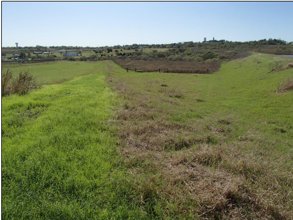
Figure 10. Disturbed zone between auxiliary spillway (on left) and earthen dam (on right). Facing southwest, toward dam outlet.
