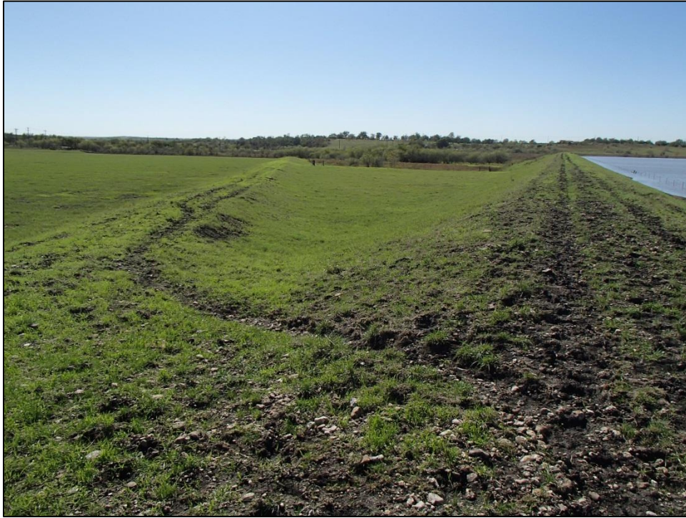
Figure 17. Disturbed zone between auxiliary spillway (on left) and earthen dam (on right). Facing southwest, toward dam outlet.
