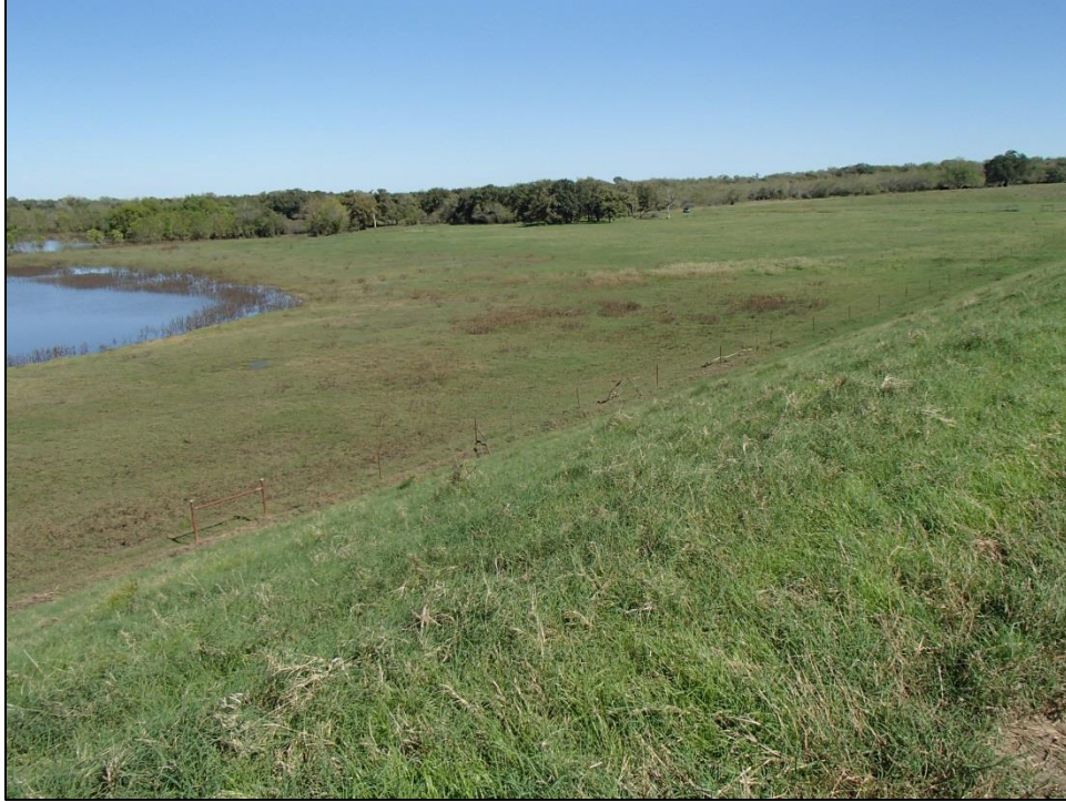
Figure 27. Devegetated area behind dam at east end, just above auxiliary spillway. Facing northeast.
