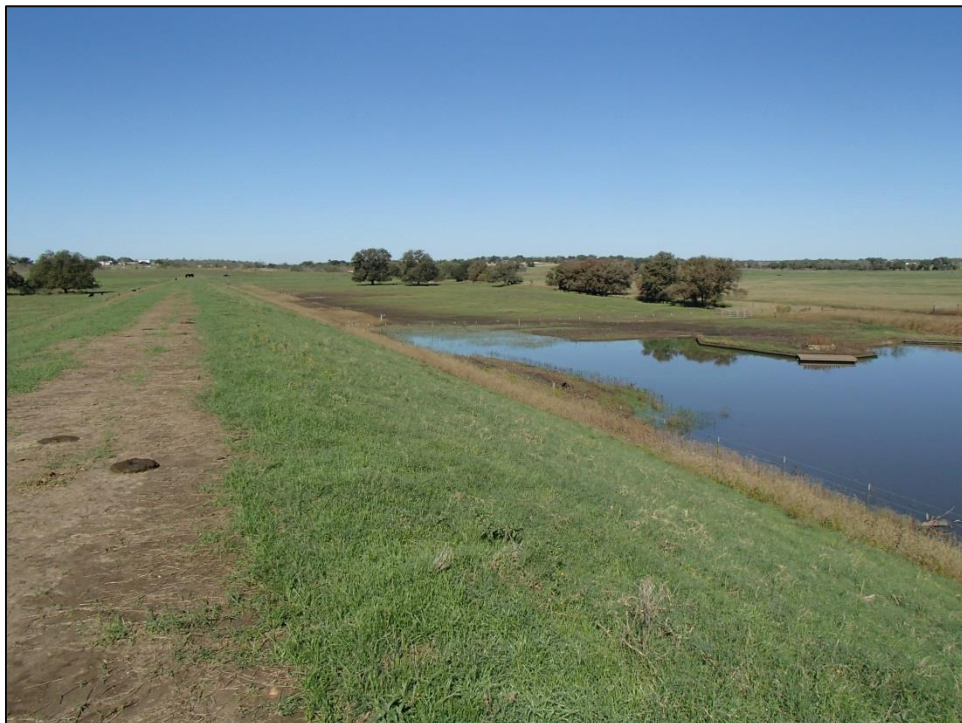
Figure 38. Earthen dam overview and periodically submerged areas next to existing pool. Facing northwest.
