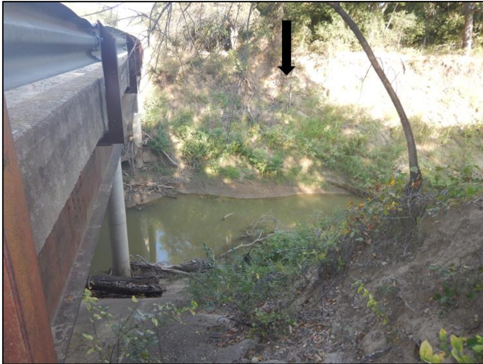
Figure 6. Overview of left bank (west side) Palo Pinto Creek; arrow indicates steel pilings from an earlier bridge crossing.
