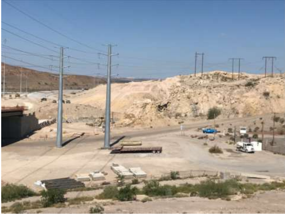
Figure 10. Recent building material dumping episode (facing northwest), note new rock wall.
