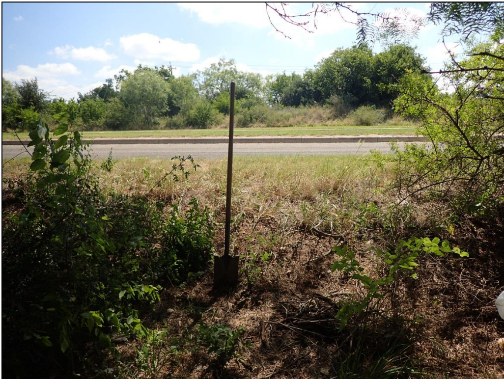
Figure 8: Showing a 2-ft high road embankment along northern end of Montgomery Road, facing east
