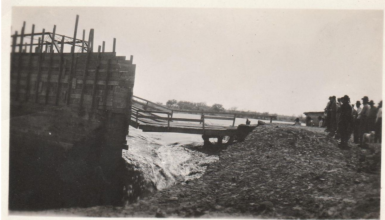
Figure 25. Flood waters damaging construction, circa 1919. Courtesy of Stephen Vinson.
