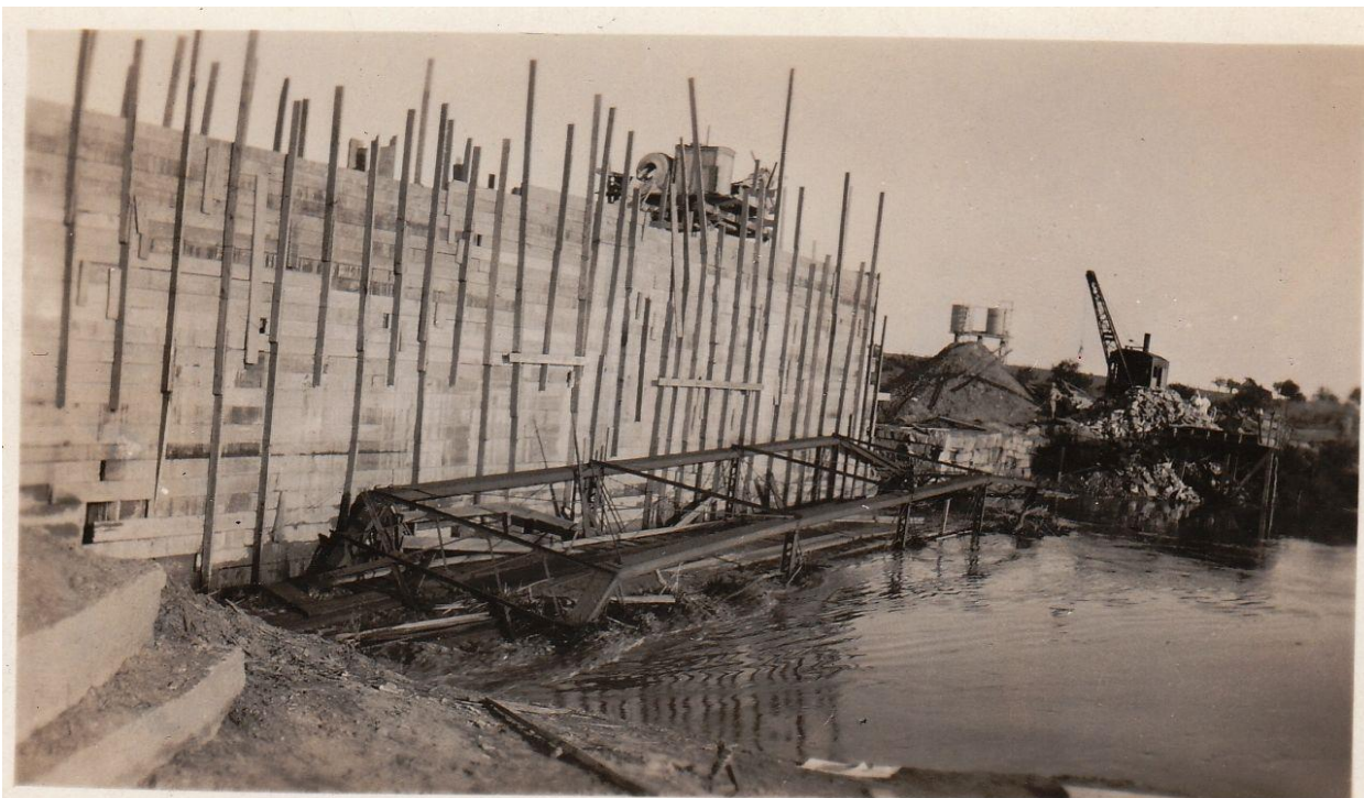
Figure 22. View of the bridge laying in the river channel. Date unknown. Courtesy of Stephen Vinson.
