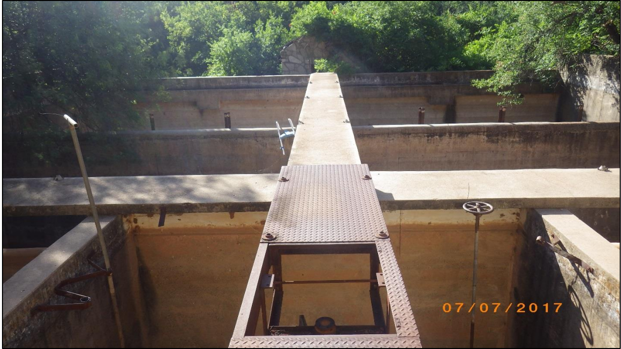
Figure 37. Intake settling basins as part of the intake structure. View is to the southeast.
