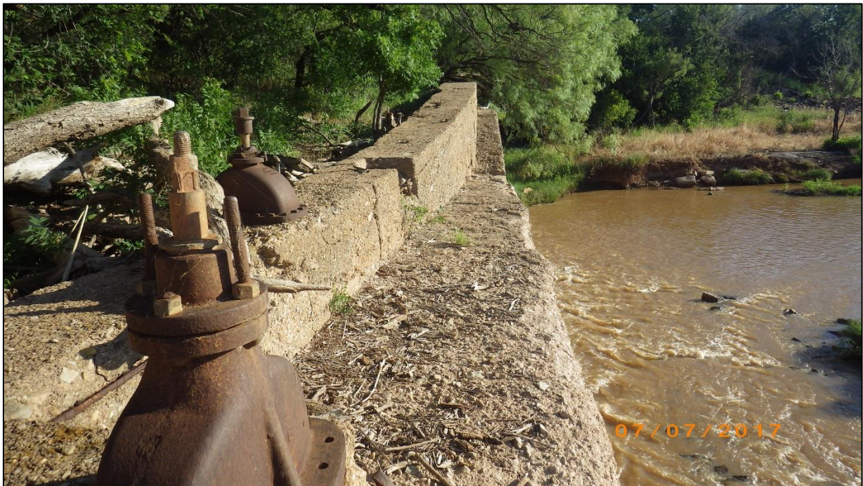
Figure 32. Overview of dam wall extending north from pumphouse. The pipeline from the pumphouse appears to be on top the dam and extends towards the intake structure.
