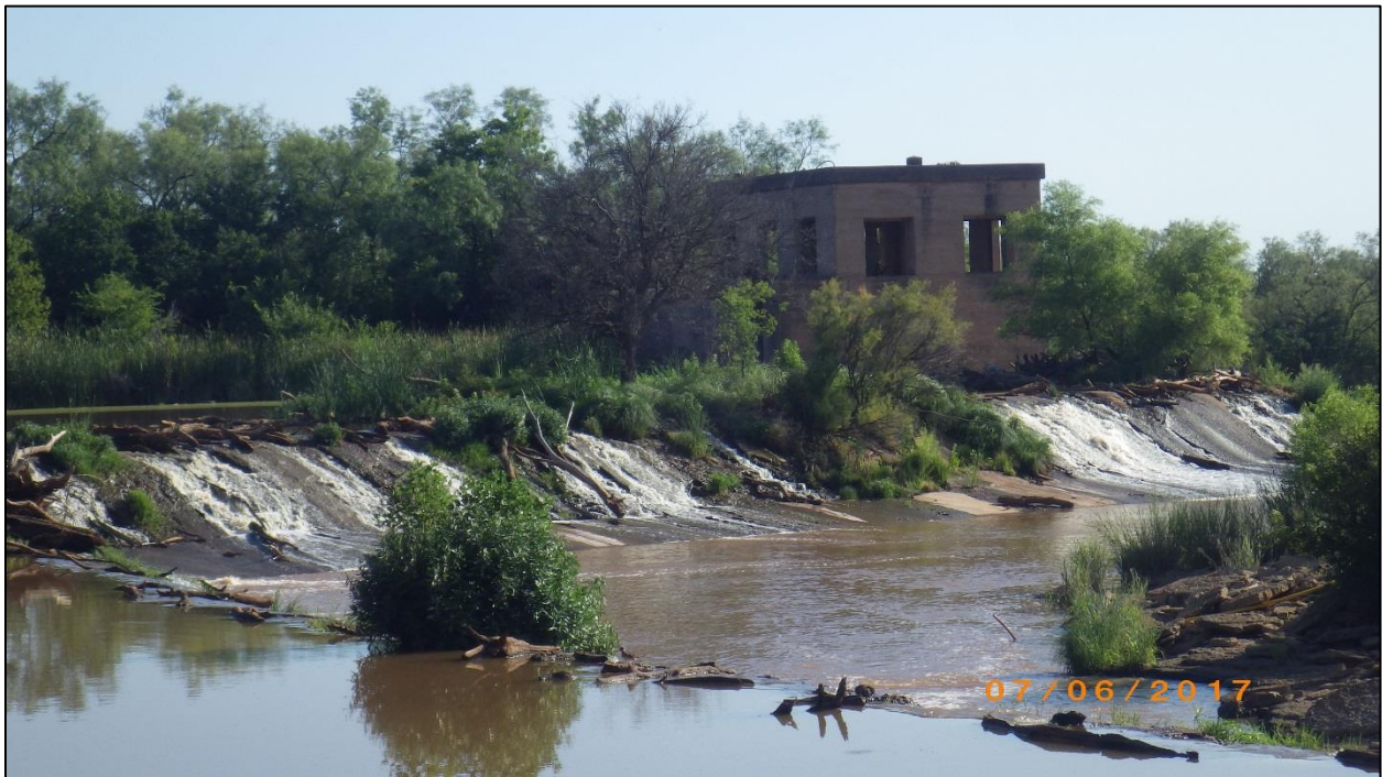
Figure 30. Overview of spillway and pumphouse from south side of river. View is to the north.
