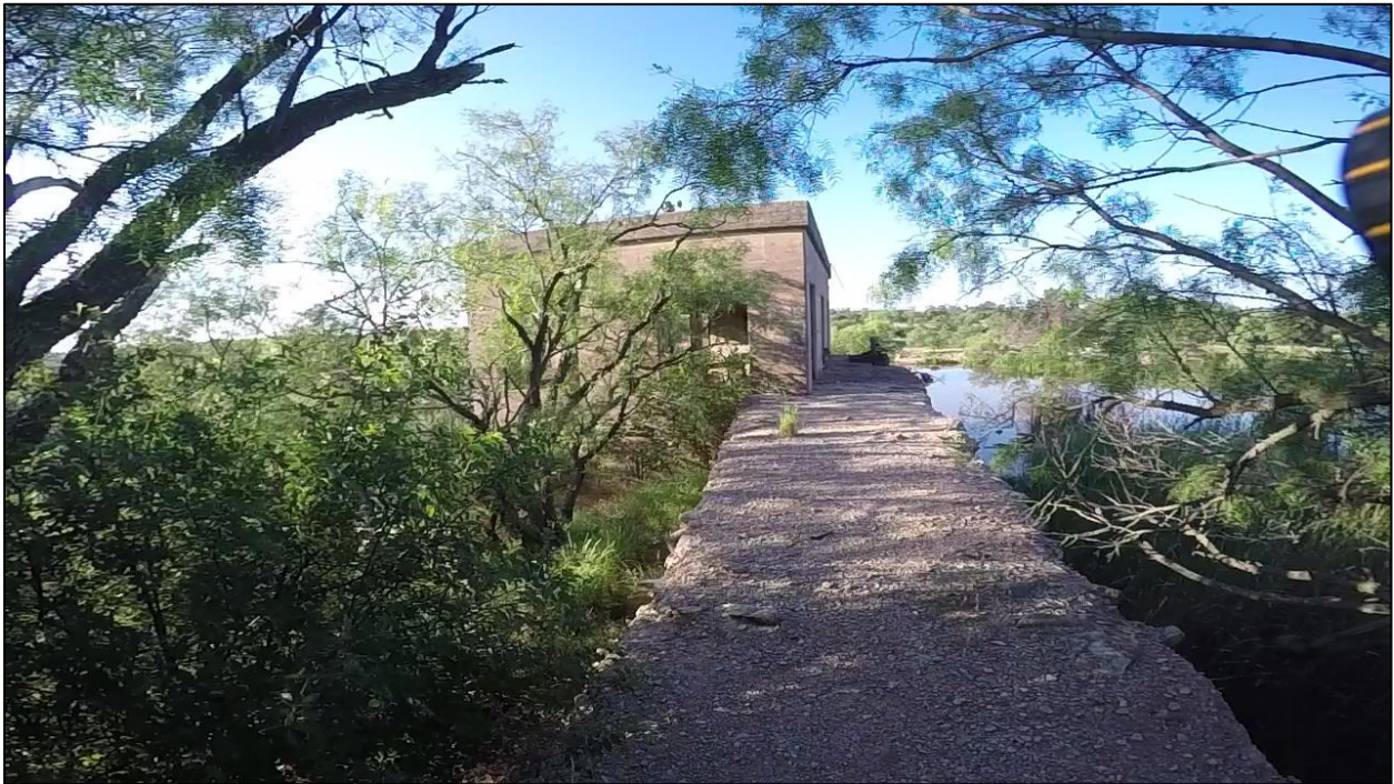
Figure 28. Overview of concrete dam where it adjoins the earthen levee, looking south out to lake and pumphouse.
