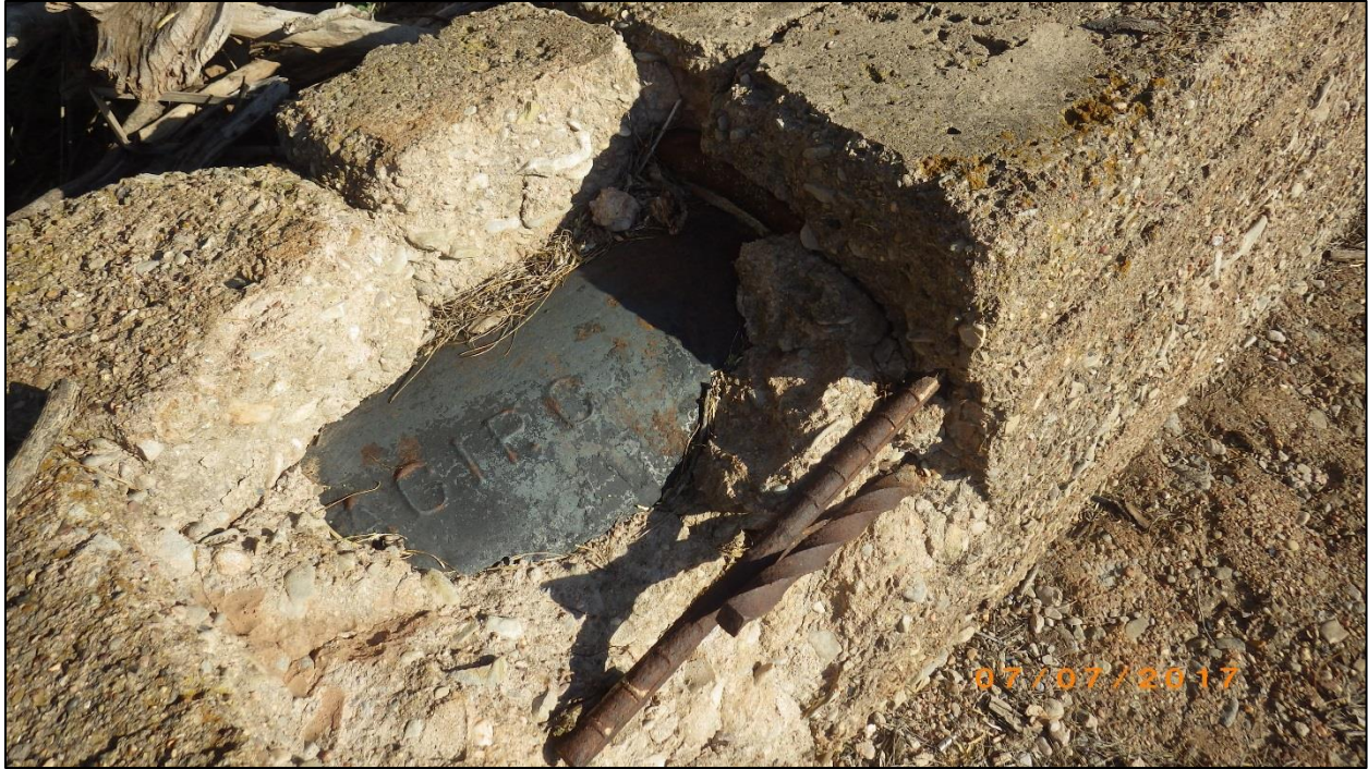
Figure 33. View of broken concrete exposing pipe and two kinds of rebar. Damascus Twist Rebar is present in the structure.
