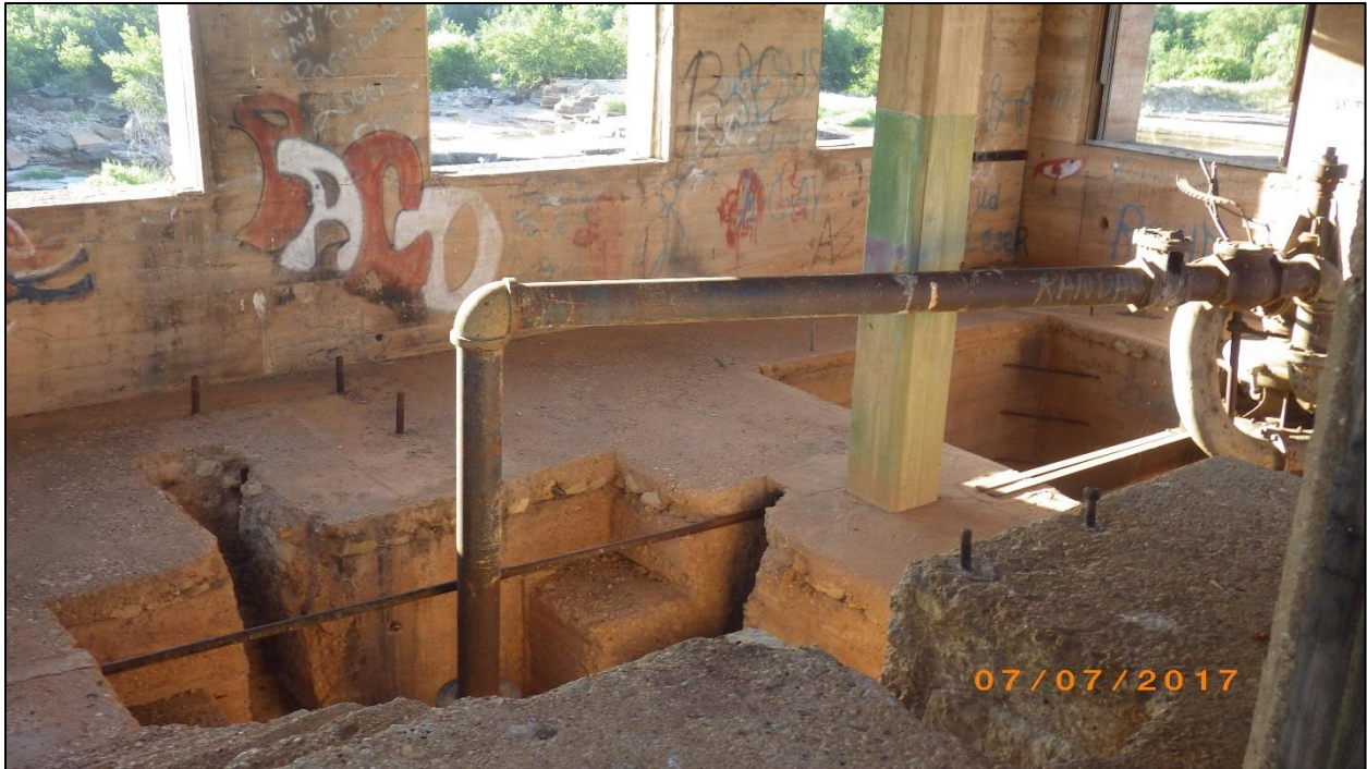
Figure 29. Interior of pumphouse. View is to the southeast.
