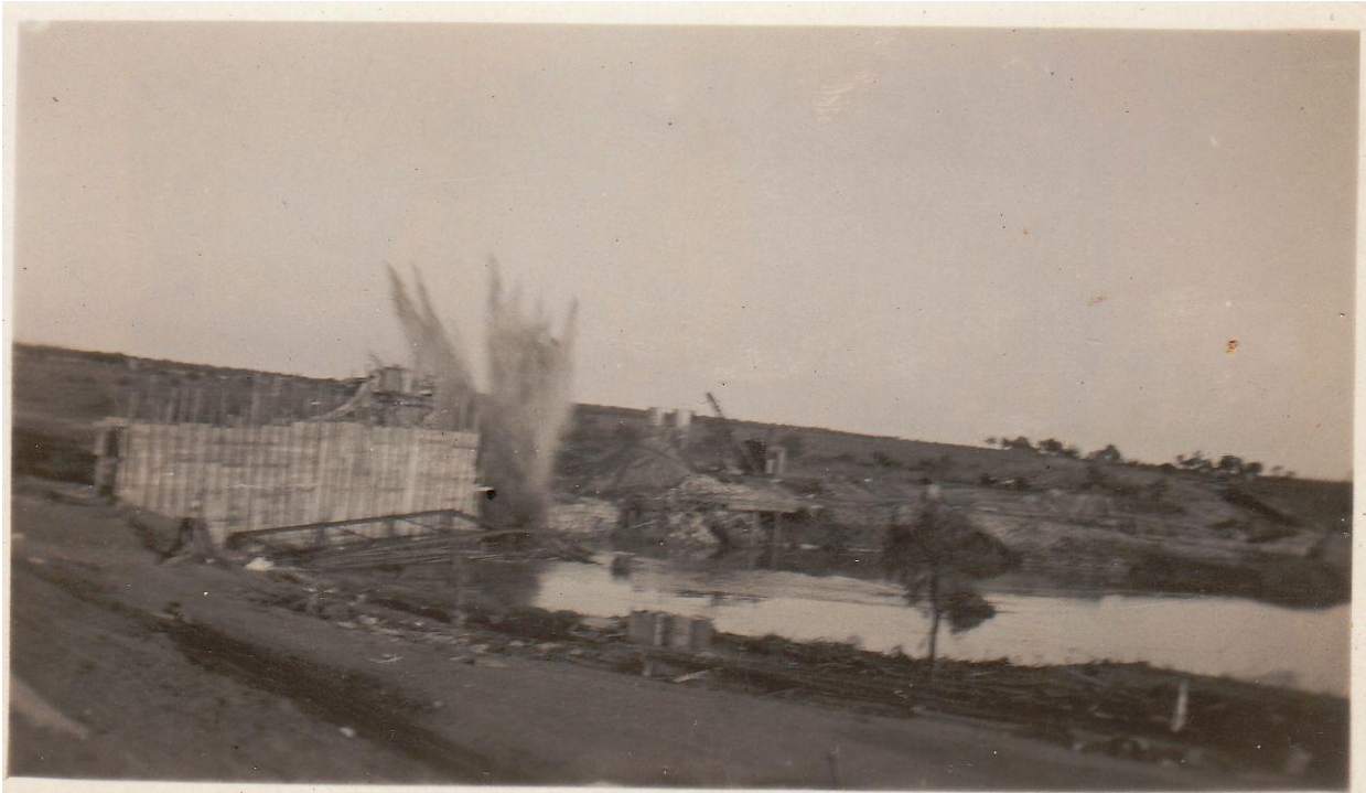
Figure 21. Blowing up southern abutment of the bridge. Date unknown. Courtesy of Stephen Vinson.
