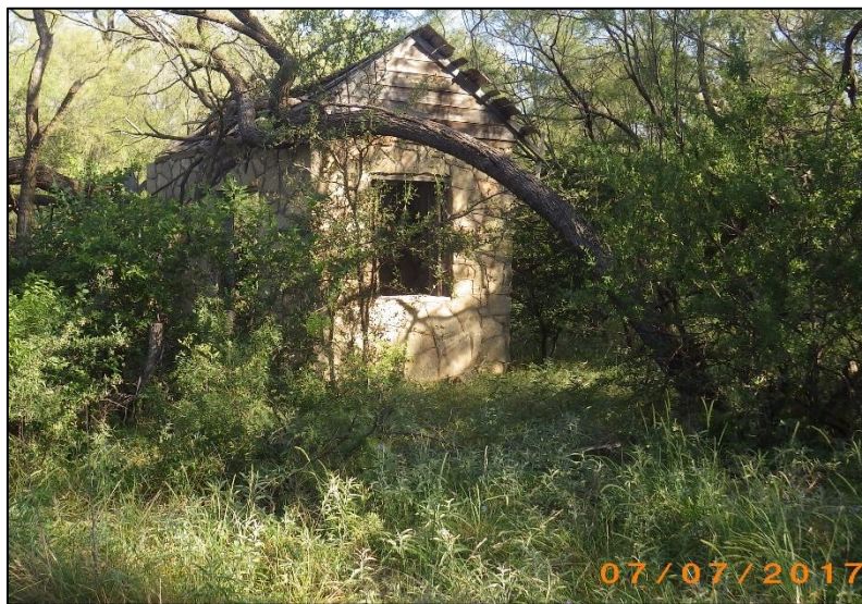
Figure 34. Small motor building northeast of intake structure. View is to the north.
