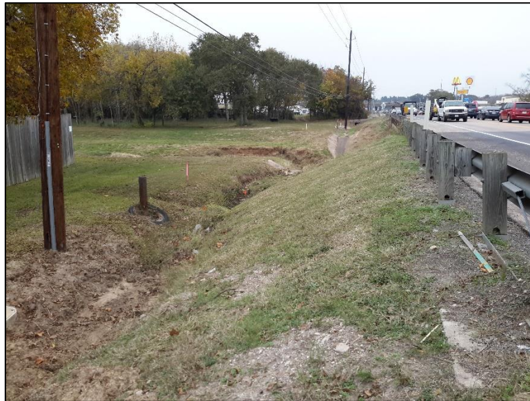
Figure 9. Willow Fork bridge crossing with extensive grading, erosion, and buried utilities; west side of FM 1463, facing northeast.
