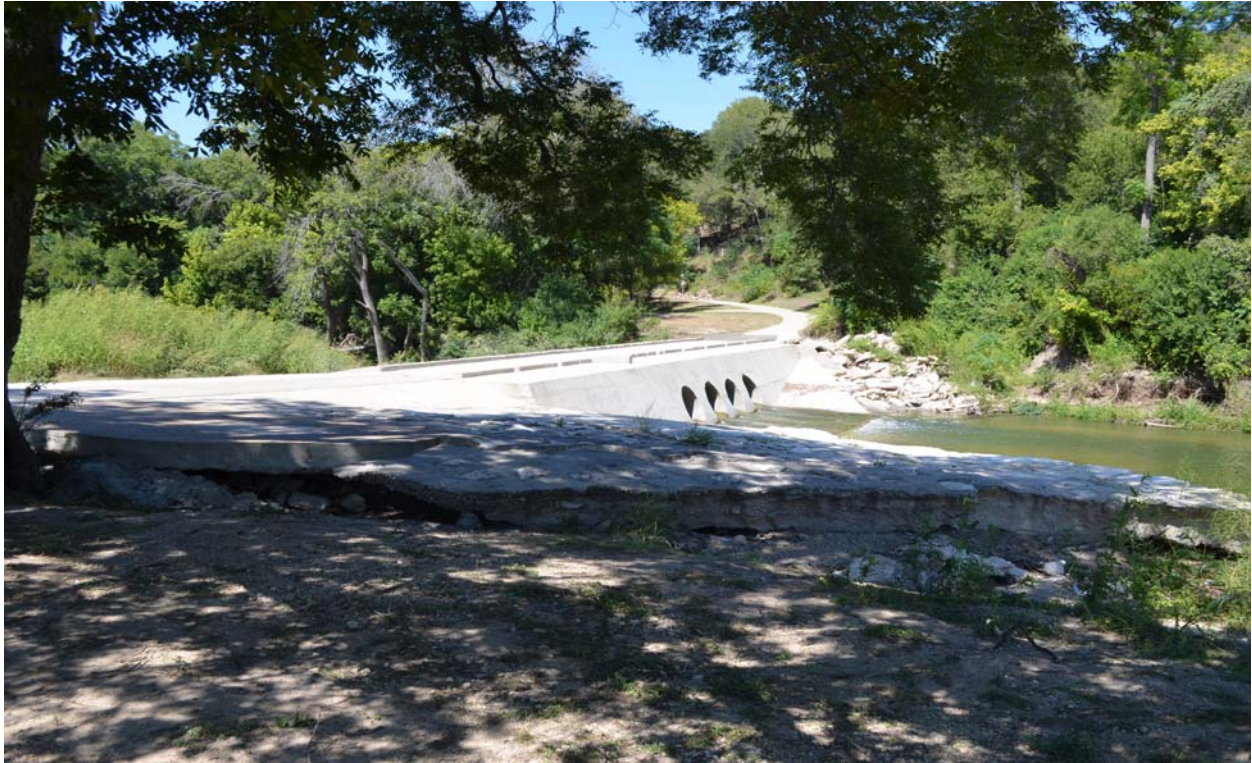
Figure 11. Northwestern view of concrete bridge at Tract 2. Note extensive erosion.
