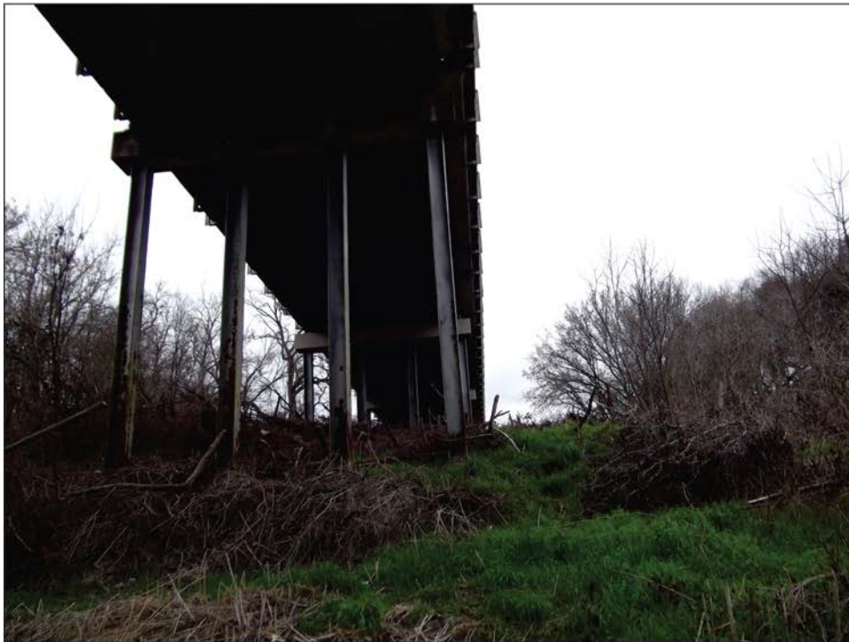
Figure 8. South abutment of existing bridge at Cowhouse Creek. Note mechanically shaped terrace.
