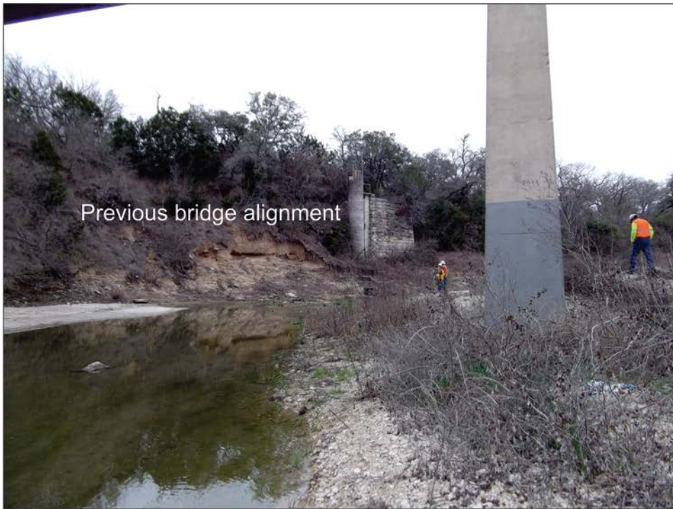
Figure 9. Existing bridge with previous alignment visible on north bank at Cowhouse Creek.
