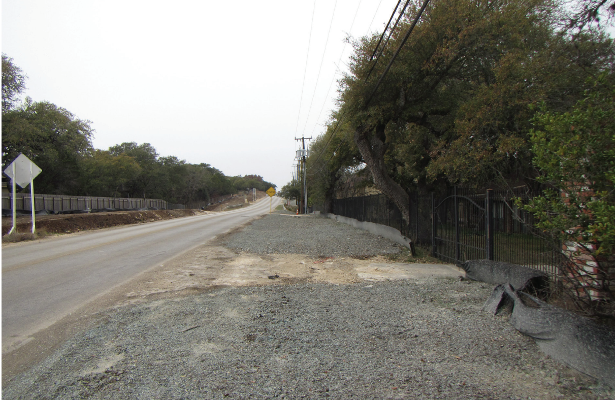
Figure 5. Photograph of grading and utilities disturbances along West Borgfeld Drive between Bonn Mountain and Wild Bloom Streets.
