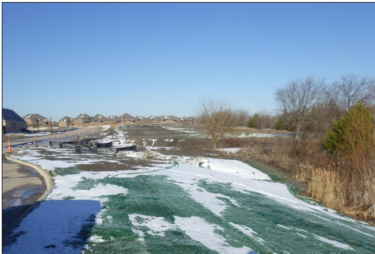
Figure 2. The southern edge of the Stone Creek Park property, facing west. Note the scraped field in the background.
