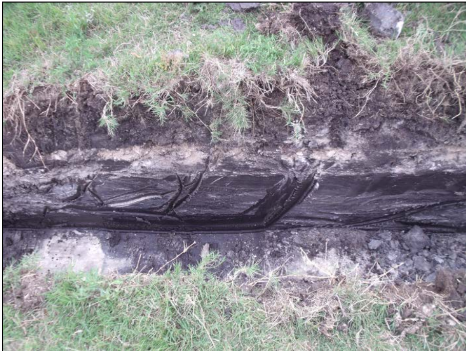
Figure 5-3. Modern top soil and road base on top of sterile dark gray clay, BHT 1.
