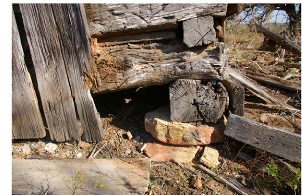
e) Detail of stone piers and hand hewn sill and floor joist.
