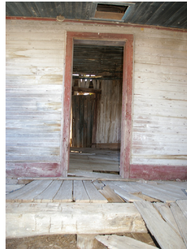
i) Detail of hand hewn sill of former porch, now supporting floor of addition.
