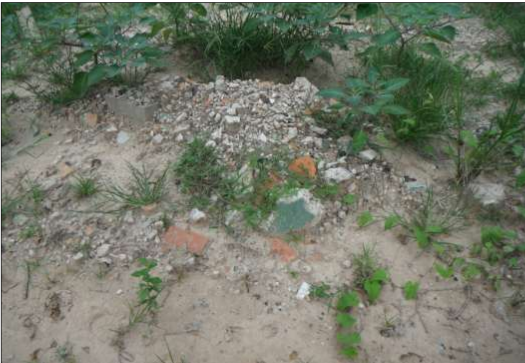
Figure 15. View of Debris Piles Surrounding Former Structure Location
