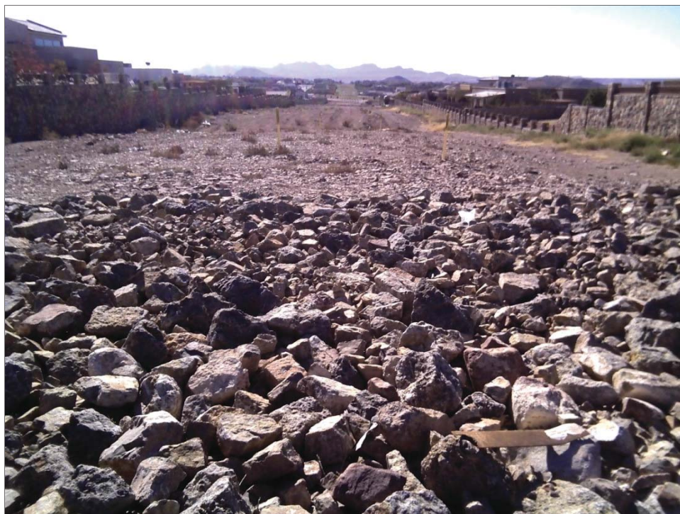
Figure 2. MP 0+0000 - Location of new pressure regulation station, facing south (Digital Roll 31122, Frame T11-6091).
