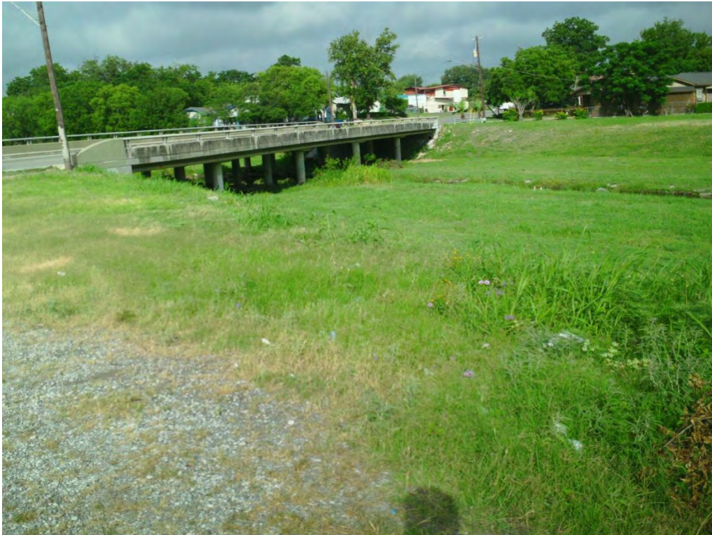
Figure 18: Overview of western terminus of proposed Martinez Creek trail facing northwest towards Cincinnati Street Bridge from STGC3.
