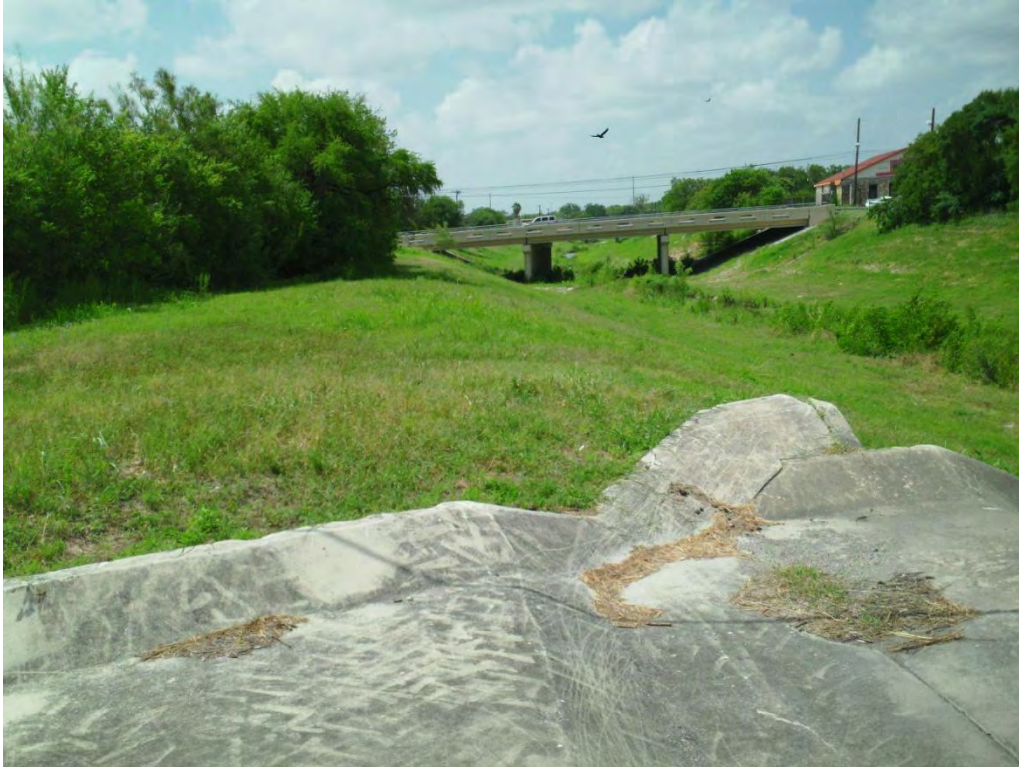
Figure 23: Overview of Project Area facing west towards Lombrano Street Bridge from drainage culvert within project area, located just north of Laurel Street towards.
