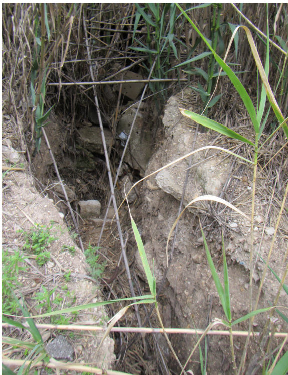
Figure 3. Erosional cut along Jefferson Street force main corridor showing dumped construction debris on the north bank of Town Creek west of Water Street.
