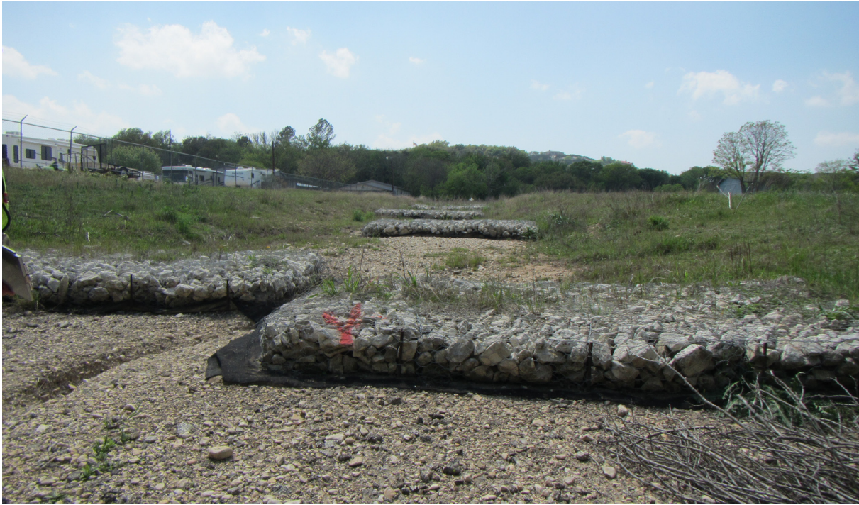
Figure 5. View to the west of the large drainage ditch at 41KR677. The site was originally recorded exposed in this drainage.
