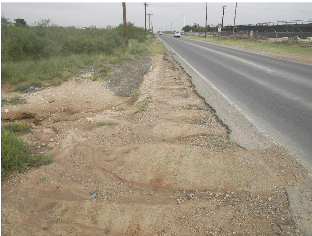
Figure 6. Erosion in right-of-way on west side of APE, looking north
