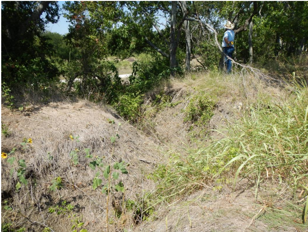
Figure 4. Erosional wash-out along the western boundary above the tributary; facing west.
