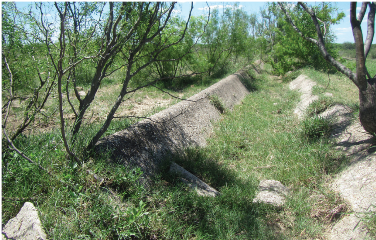
Figure 5. Photograph of dilapidated concrete-lined irrigation ditch on the heavily modified floodplain of Elm Creek.
