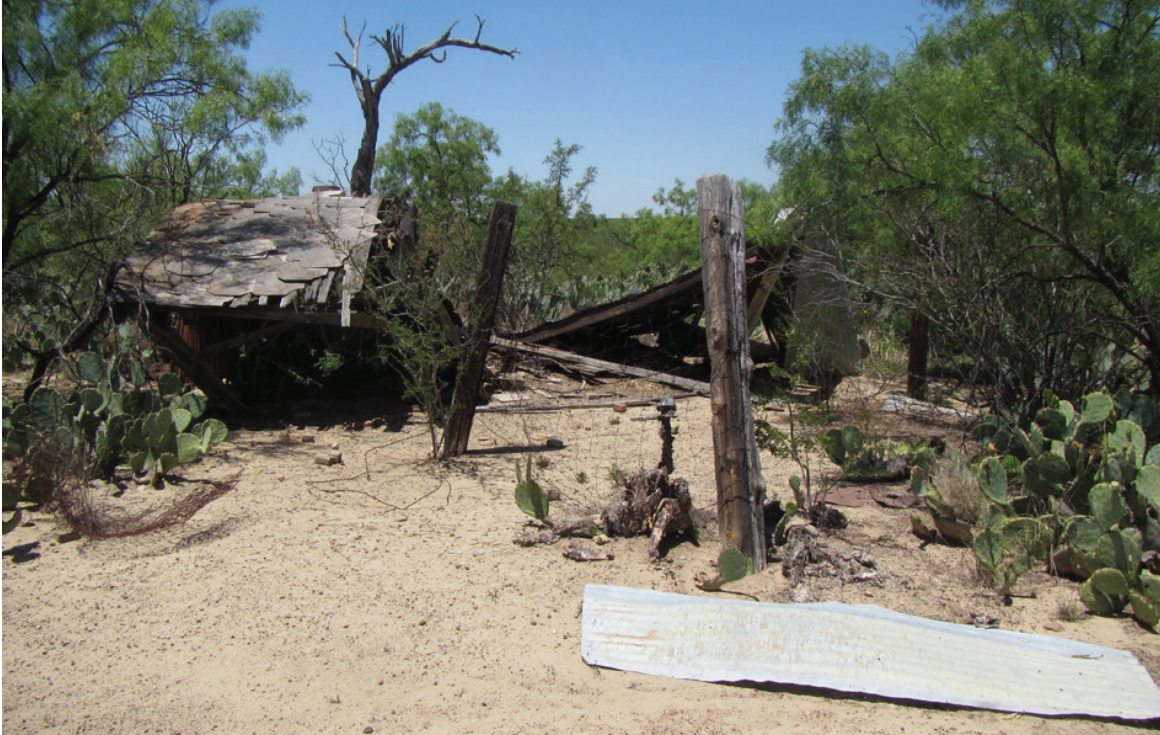
Figure 14. Photograph of one of the two ruinous wood-frame outbuildings at 41MV389.
