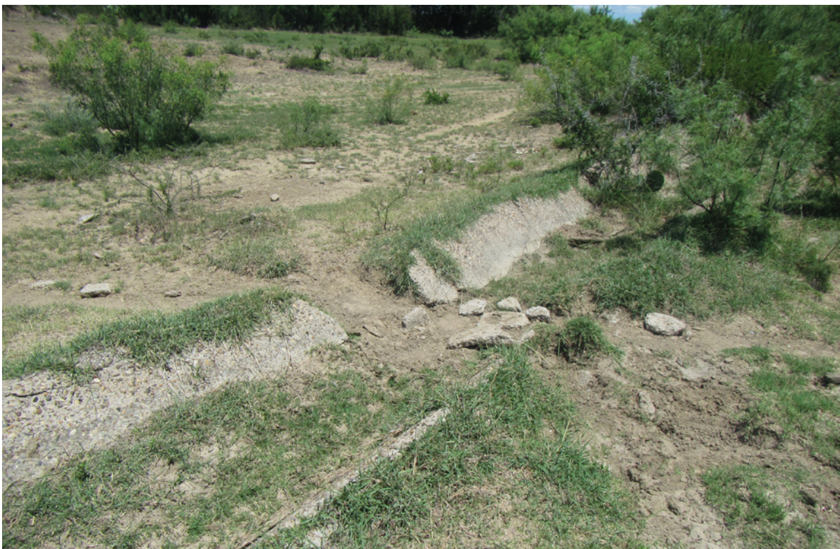
Figure 34. Photograph of lateral ditch in the Kincaid irrigation system incapacitated by broken concrete.
