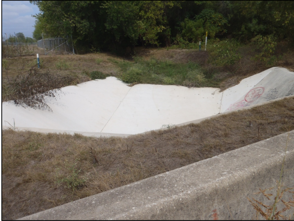
Figure 5. Prior disturbances within Survey Area 2, including a concrete-lined drainage structure and underground water lines, facing northeast.
