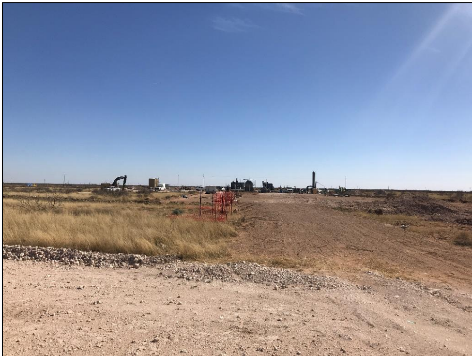
Figure 7. General overview of the APE, facing south along the proposed pipeline trench from the north tie-in.
