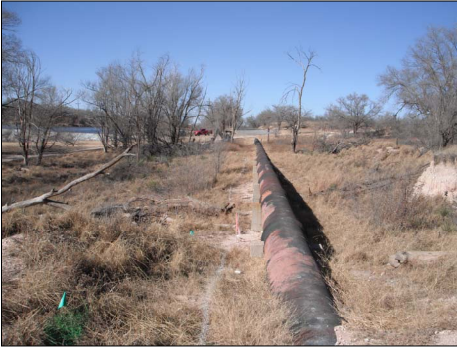
Photo 2. Setting for Trench 1 and Trench 3, at proposed location of Segment 1 (parallel to existing line), facing north.
