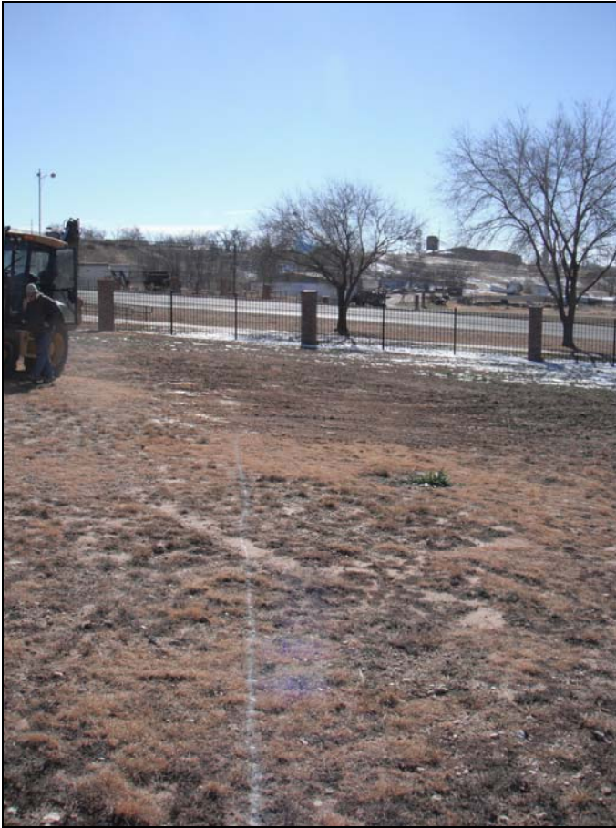
Photo 7. Setting for Trench 18 at north end of proposed location of Segment 4, facing southeast.
