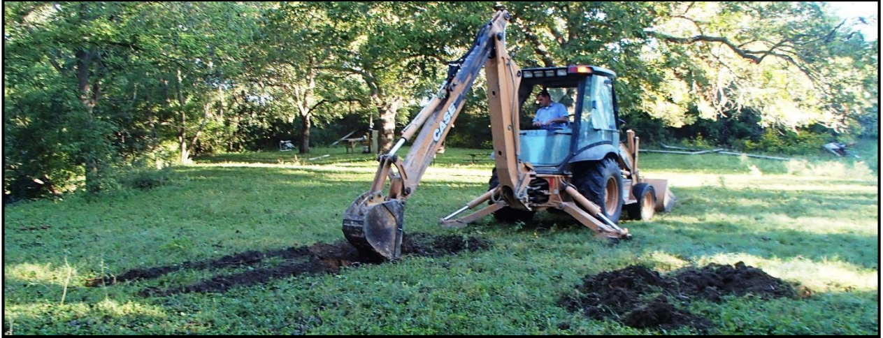
Figure 6-10. Overview of Backhoe Trench 3 location on low Terrace ( T_1 ) with picnic area in background. Note the proposed outfall is to the left of picture.
