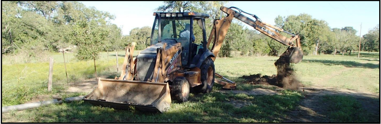
Figure 6-2. Backhoe Trench 1 location on upper terrace (T 3 ), view north with existing sewer line in open area in left background.
