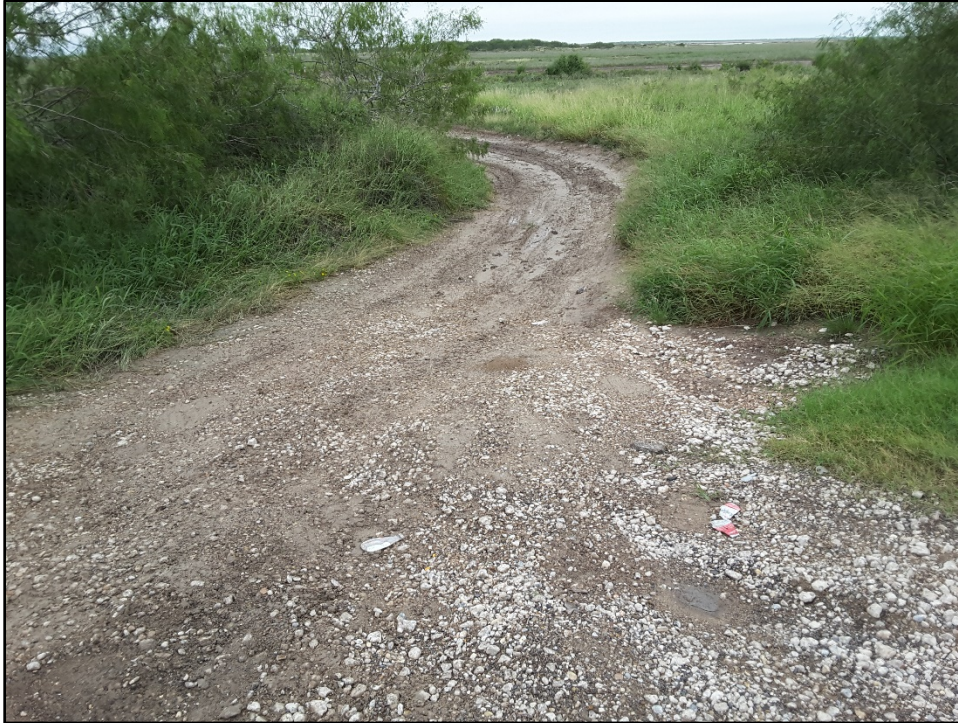
Figure 13. Existing access road on tract ND-CAM-082.000 disturbed by previous pipeline construction, facing south.
