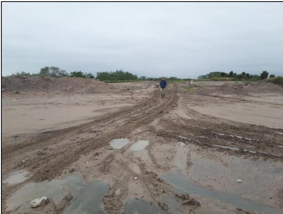
Figure 12. Existing access road on tract ND-CAM-082.000, facing north. Access road has long been in use for existing collocated pipeline marked by orange and white posts in background. Note wide road cut through low lomas near surveyor.
