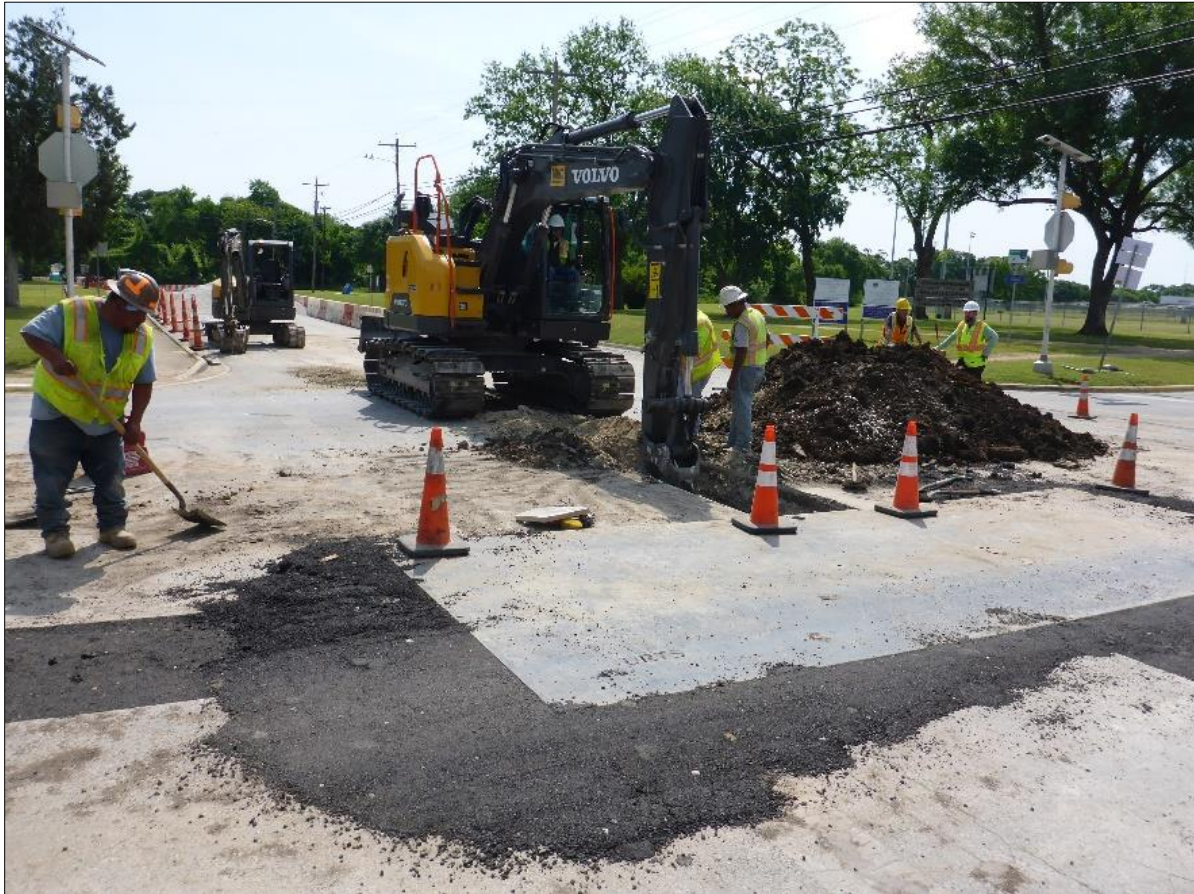
Figure 9. West end of waterline trench, taken on April 27 th . The fresh asphalt is covering trenches outside the area of potential effects (APE).
