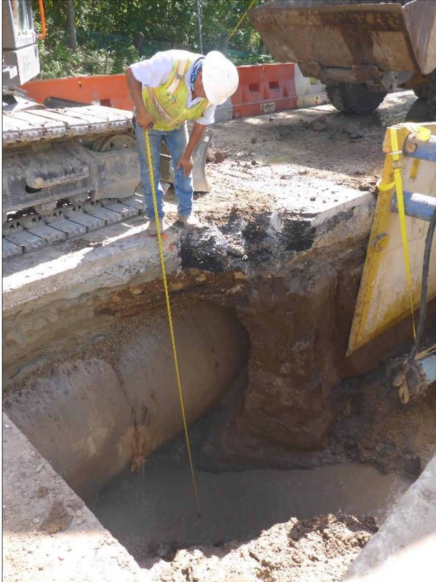
Figure 23. Expansion of Entry Trench #2 underway, with leaking storm pipe on left, on October 4 th .
