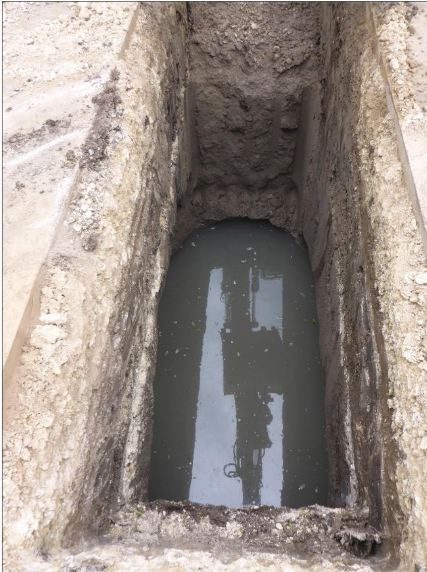
Figure 11. The Drill Rescue Trench on April 30 th .
