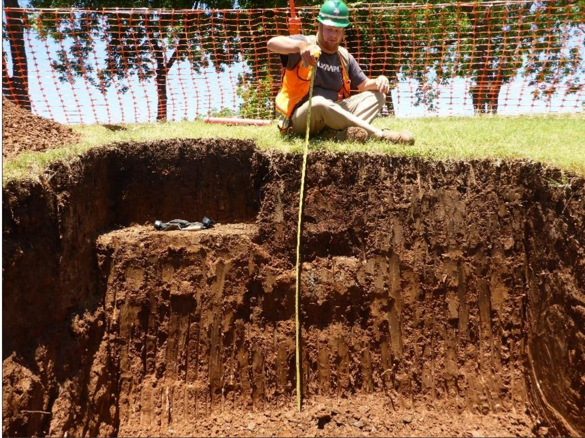
Figure 19. Manhole Access Box excavation on May 17 th , with the remnants of a one-meter excavation unit in top left of trench.
