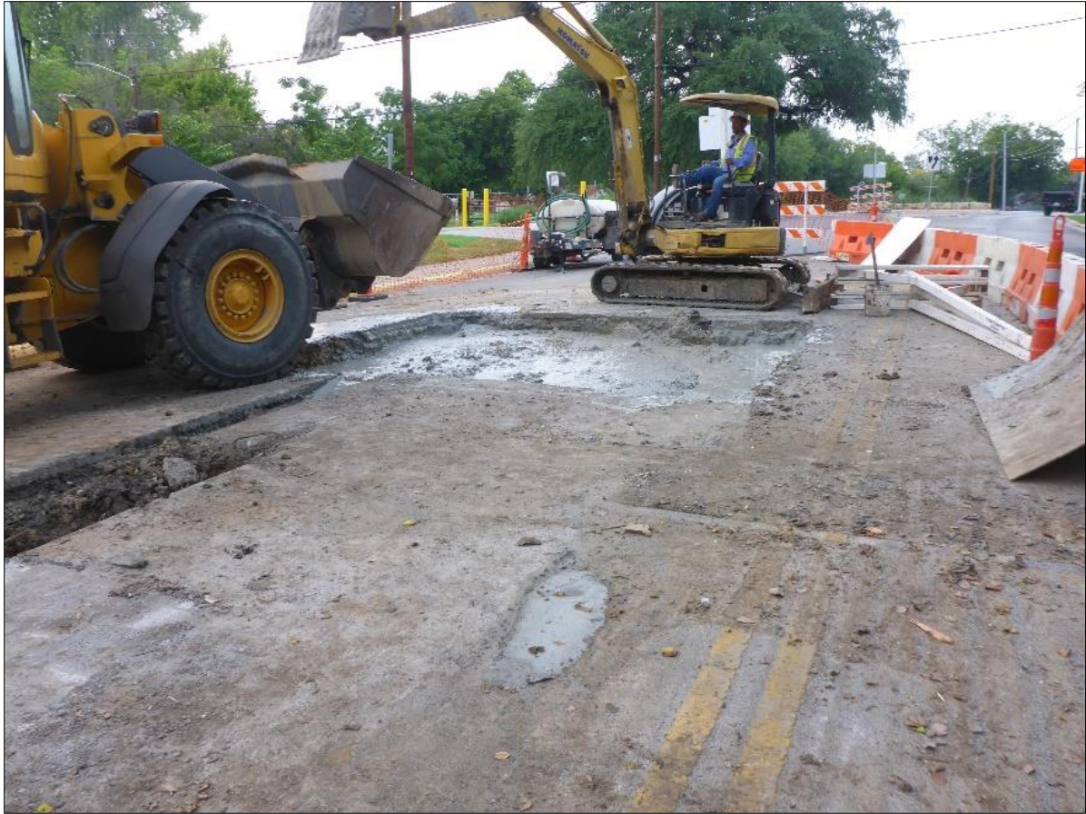
Figure 21. Shallow “dead man pit” at east end of Entry Trench #2, taken October 3 rd .
