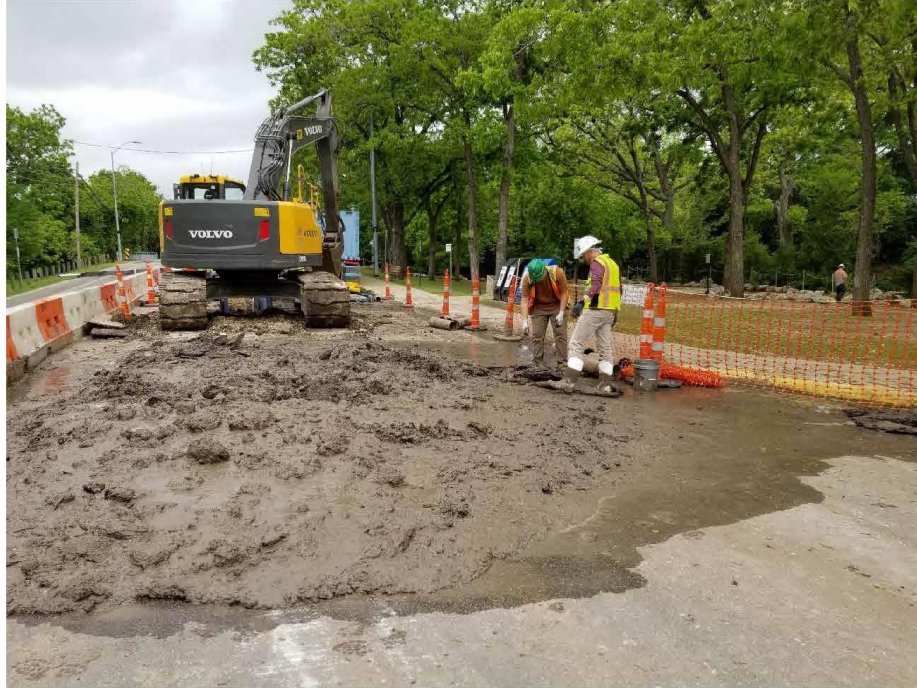
Figure 8. Highly saturated back dirt pile.
