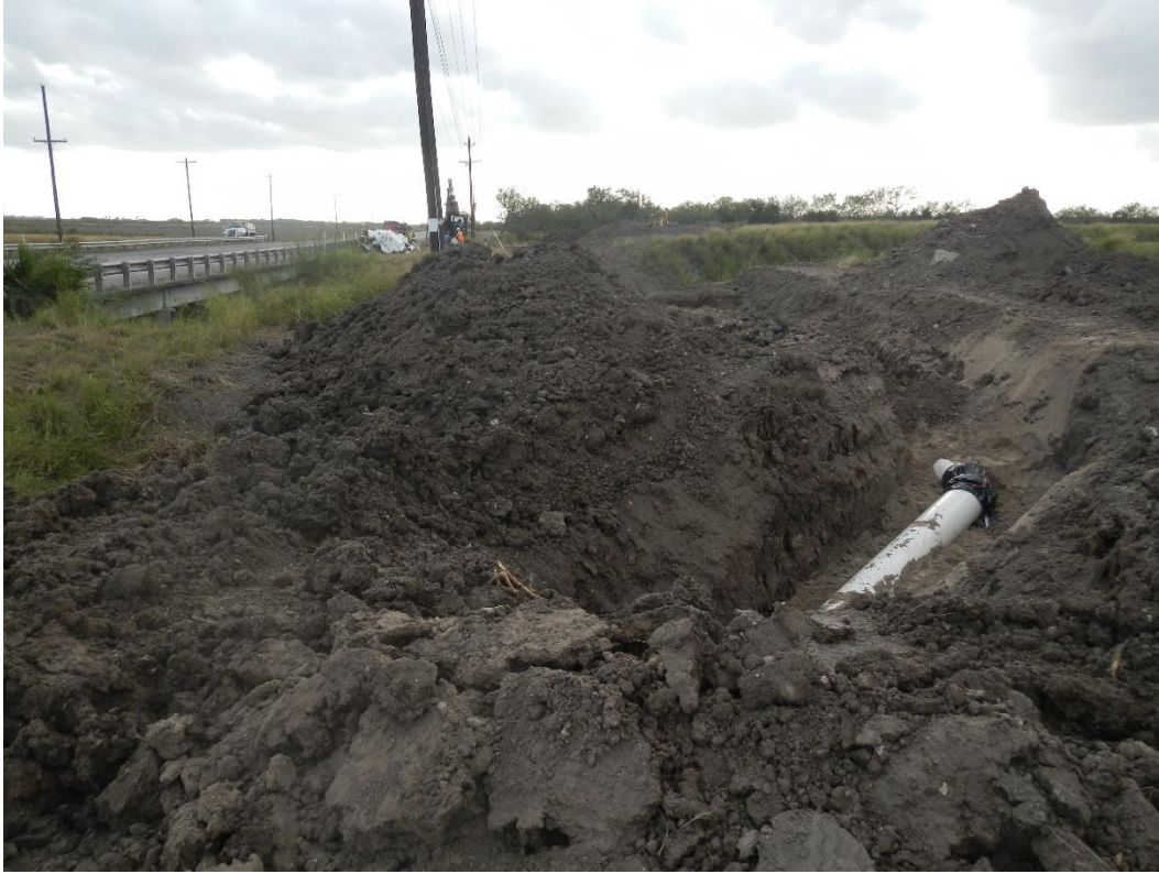
Figure 6. Subsurface utility disturbance
