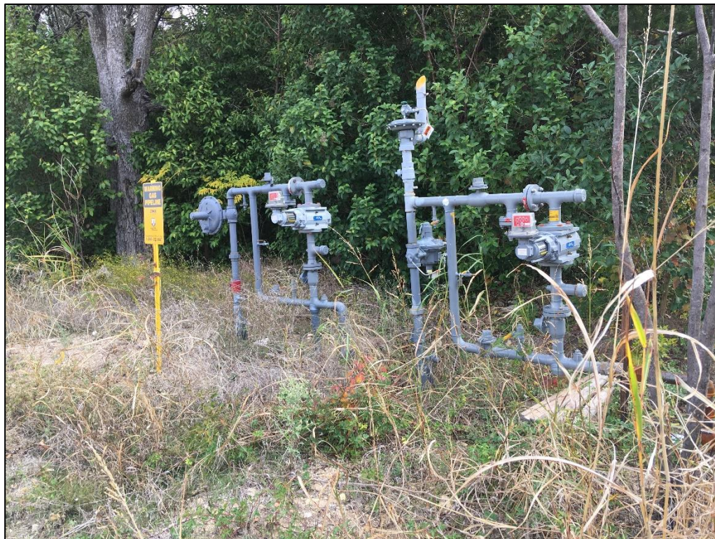
Photo 18. Northern portion of project area. Station for buried gas line. View to the northeast.
