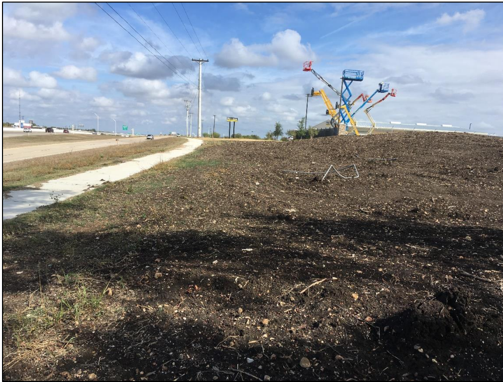
Photo 21. Northern portion of project area. Note disturbances from construction activities. View to the northeast.
