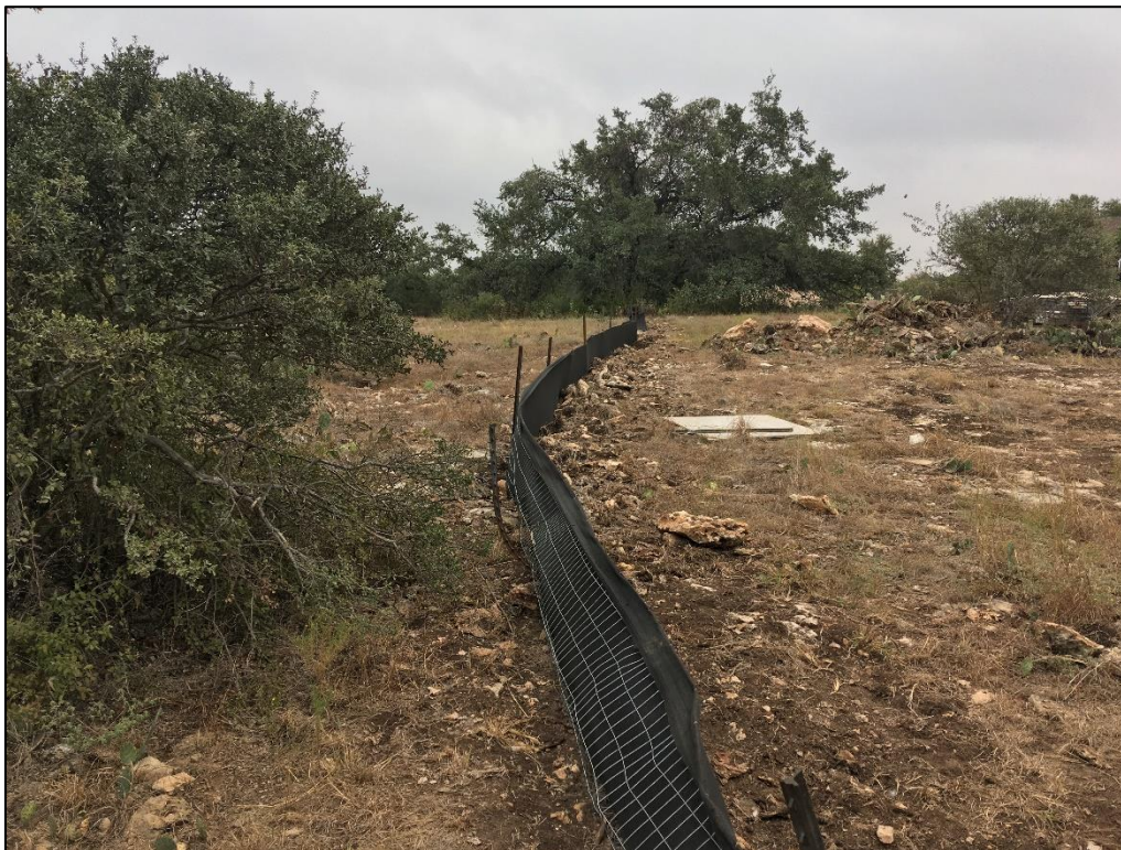
Photo 7. Southern project boundary. Note silt fencing and disturbances on the right side of photo from construction of a housing development south of the project area. View to the east.
