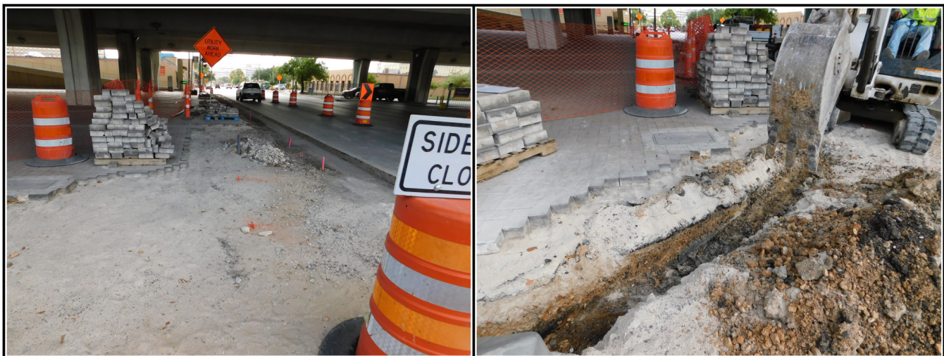
Figure 6-3. The image on the left shows the layout of the trench under the Pan Am Expressway. The image on the right shows the profile of the northern trench wall.
